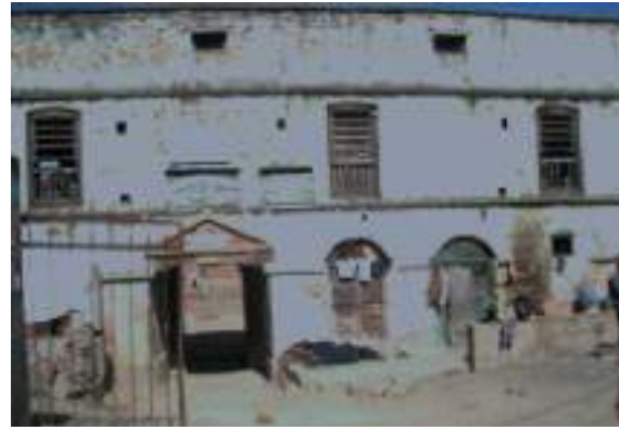
Substandard Structures Photo credit: EMI, 2008
