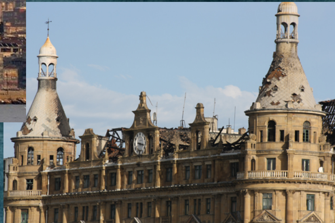
Fire in Istanbul's Historic Haydarpaşa Train Station, 28 November 2010
