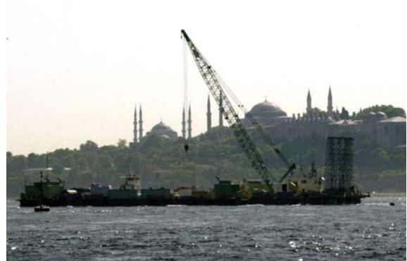
Building of a railway tunnel underneath the Bosphorus connecting the European and Asian continents
