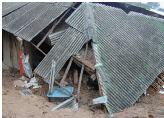
<Damaged House by Landslide in 2003> - Samcheok City, Gangwon Province -
