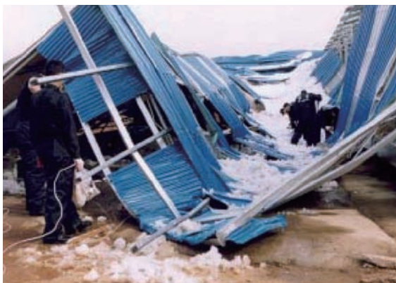
<Cattle Shed Damaged by Blizzard in 2004> - Nonsan City, Chungnam Province -
