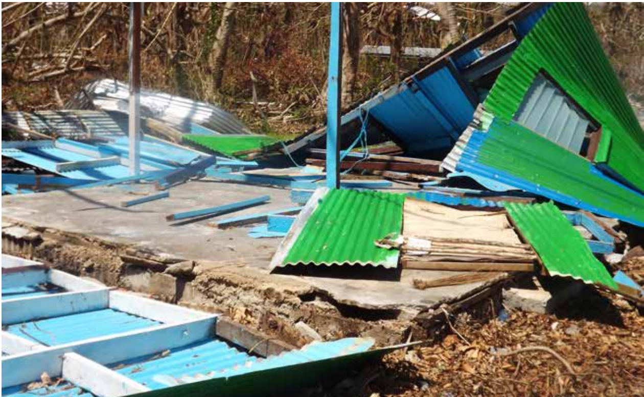
> One of the Manua School buildings after Cyclone Pam. Photo: Save the Children
