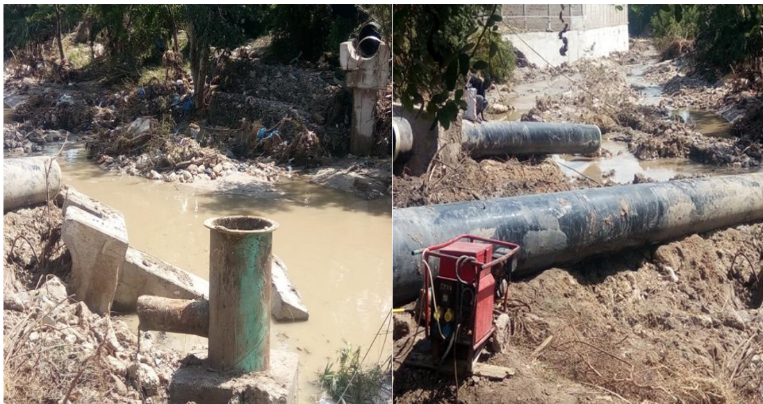
Plate 1 Water transmission (30" diameter) dragged away by flooding water across Mbezi river in October 2017
