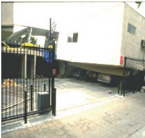
Figure 12 Soft Story Building Collapse
