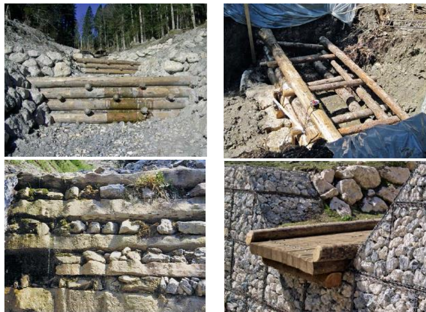
Top: Small wooden check dams, Bottom: Small stone check dams, the right one with a metal gabion mesh (Rimböck, Höhne, Mayer, & Wolter-Krautblatter, 2015)
