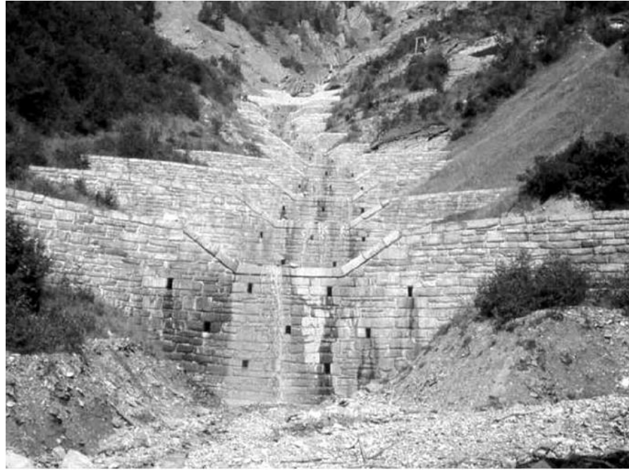
Transverse toe slope stabilization, Austria (Jakob & Hungr, 2005)
