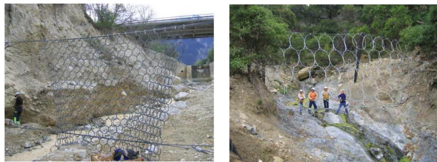
Left: Pulling up of a ring net during installation; Right: Alternative mesh size at Gaviota Pass, Canada (Wendeler, 2016)
