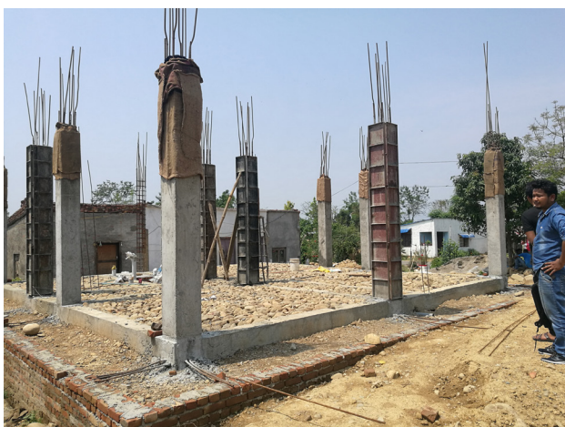
Chitwan: RCC frame structure under construction. The home owner has applied for the second tranche of the housing reconstruction grant and the application has been forwarded to the municipality.
