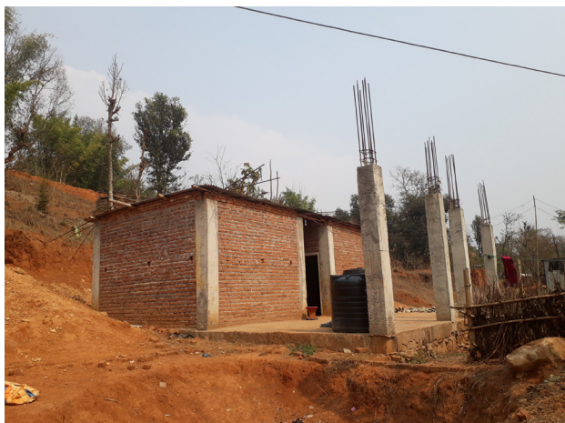
Bhanu Municipality, ward-2, Tanahun: house reconstructed with RCC structure but due to road right of way conflict and formation of new municipality and its building requirements he home owner is not allowed to construct rigid floor and even they constructed RC frame structure beneficiaries were living by putting CGI roofs and brick infill walls.
