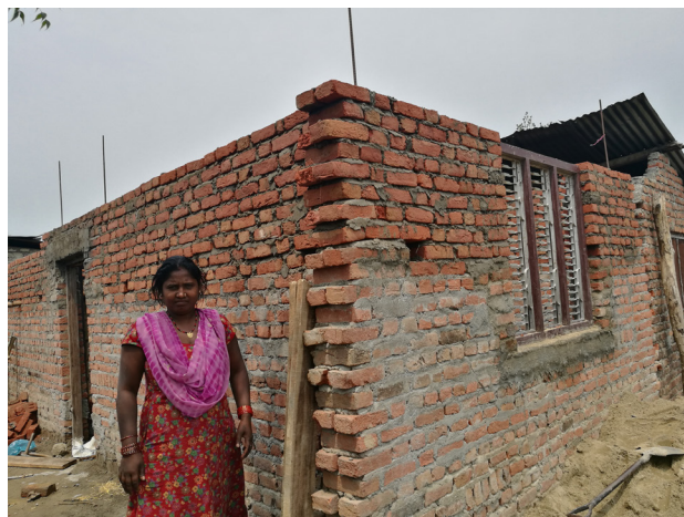
Sunawal 2, Mukhiya Tole, Parasi: the home owner has received the 2nd tranche but vertical and horizontal reinforcement has not been properly implemented and so the house has not been recommended for the third tranche. During the visit the DLPIU sub-engineer said they had been providing regular follow up to the household but the home owner has not been willing to follow the guidelines and their suggestions.
