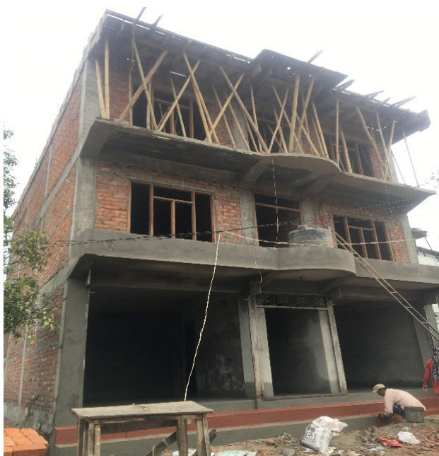
Khandbari Municipality, ward-8, Sankhuwasabha: RCC frame structure with 998 sq. ft. plinth area, and 16 nos 12" *12" Columns. The house is 3 storeys with underground. The NRA, Building DLPIU engineers are confused about whether it is compliant or not but the structure has been approved by the municipality office.
