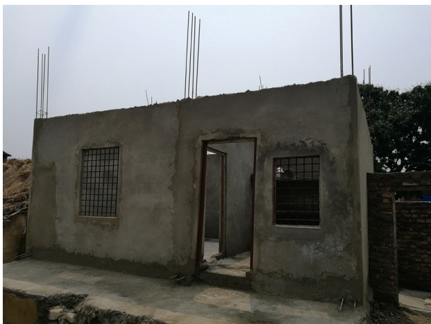
Sunawal 9, Bankattiya, Parasi: RCC frame structure house under construction. As per the comments from the DLPIU engineers during the visit the house will be eligible for next tranche immediately after the roofing is completed (third tranche does not require roof to be released).
