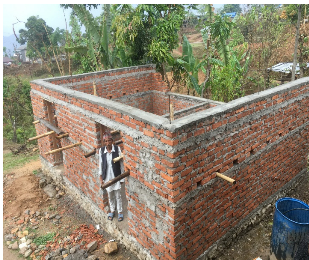
Khandbari Municipality ward-8, Sankhuwasabha: a brick and mud mortar masonry house with RC banding under construction. This house is being constructed under the supervision of NRA field engineer with the help of trained masons. The beneficiary has received the first tranche and is waiting for the second tranche. The house is considered compliant so they should receive the second tranche.
