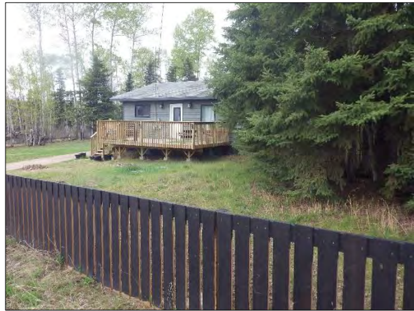
Combustible Un-Skirted Decking
