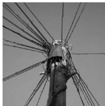
Figure 5. Network Links - Copper Telephone Cables (bottom) and Microwave Dish for a point-to-point link (top)
