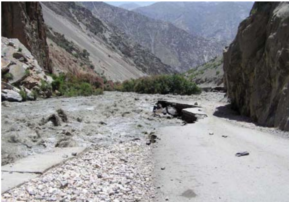
Figure 6: Damage to highway by a flash flood in July 2005 in Garam Chasma, Chitral, Pakistan
