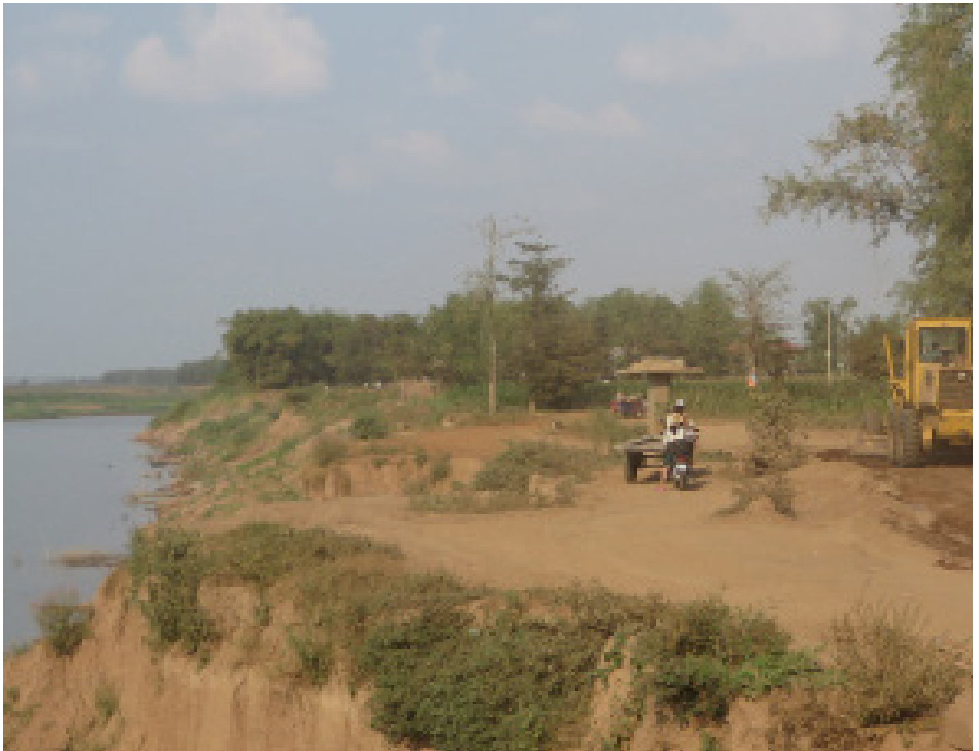
Figure 10: Road destroyed by landslide in Roka Thom, Kampong Cham, being rebuilt by local authorities.
