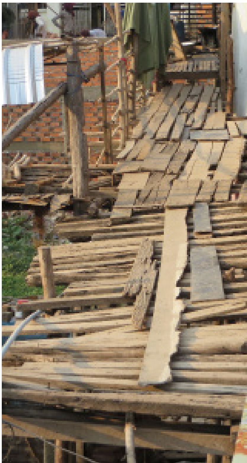
Figure 24: Insecure walkway, 2-3 m above ground.
