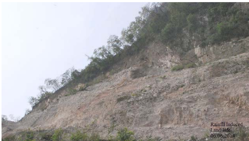
Rainfall induced Landslide, Uttarakhand, June 6, 2014.
