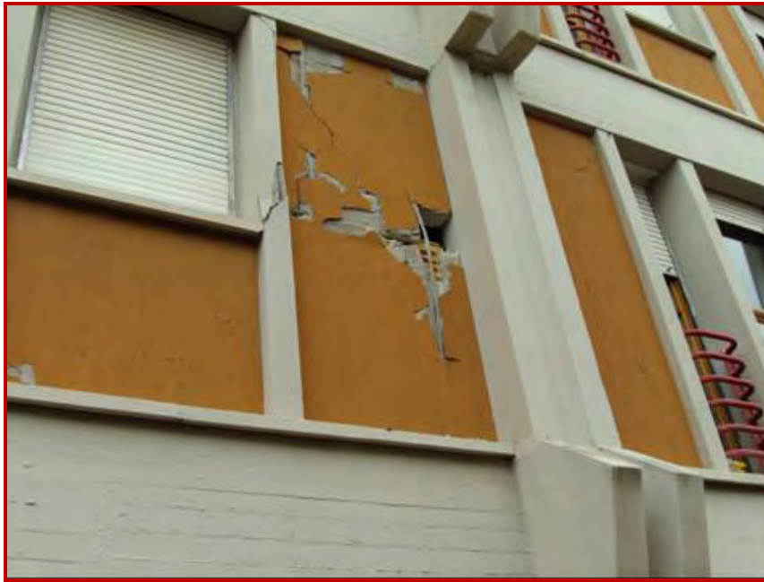
Figure 45. Detail of reinforcement of an infill wall by means of steel strips
