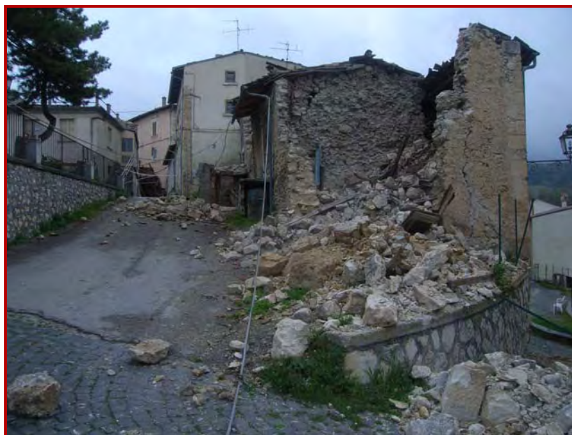
Figure 20: Collapsed masonry structure
