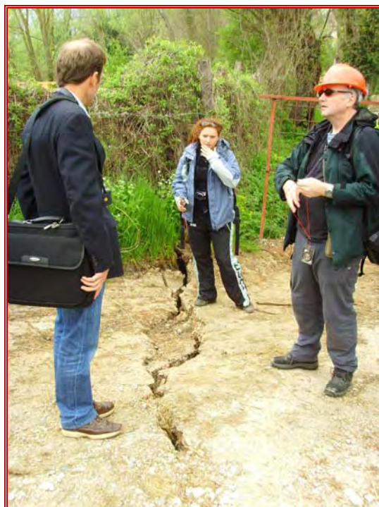
Figure 60: Tension cracks on the abutment adjacent to the bridge at Madonna Del Ponte
