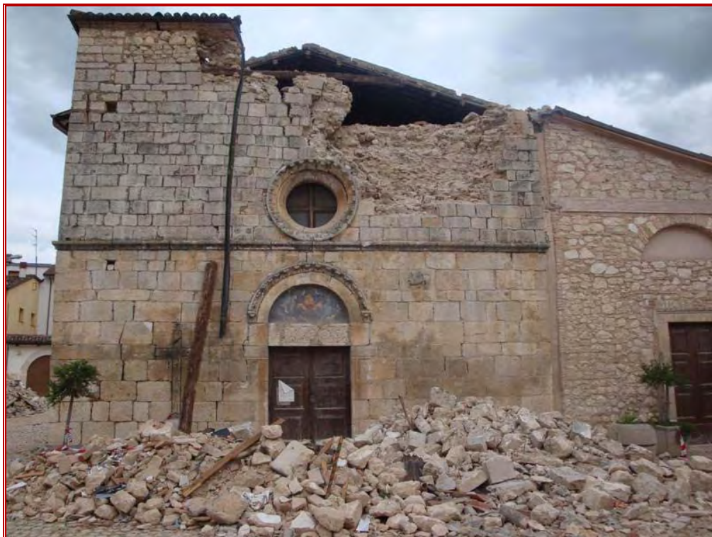
Figure 15: View of very heavy damage to church with wall failure and partial collapse of roof.
