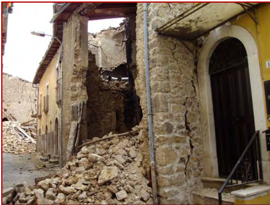
Figure 22. Example of masonry building damage in San Gregorio.
