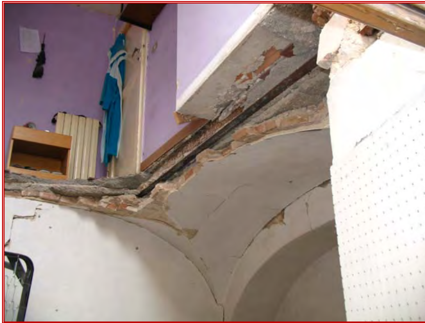
Figure 39: Example of collapse of vaulted floor in L'Aquila
