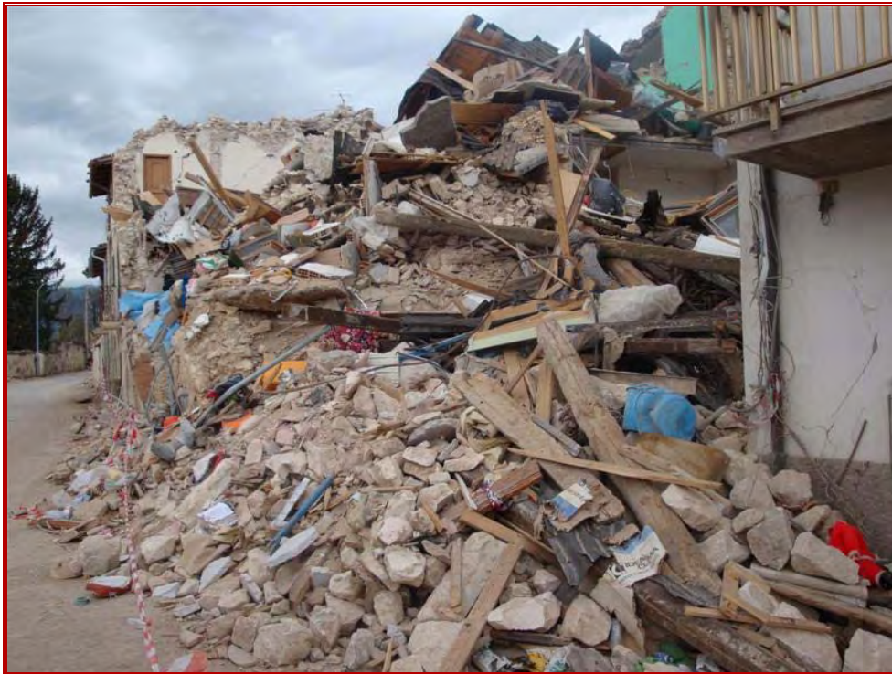
Figure 14: View of total collapse (Grade 5) of masonry building showing composite nature of building materials.
