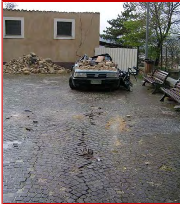
Figure 53: Tension cracks passing through stone paving and single storey building at Paganica
