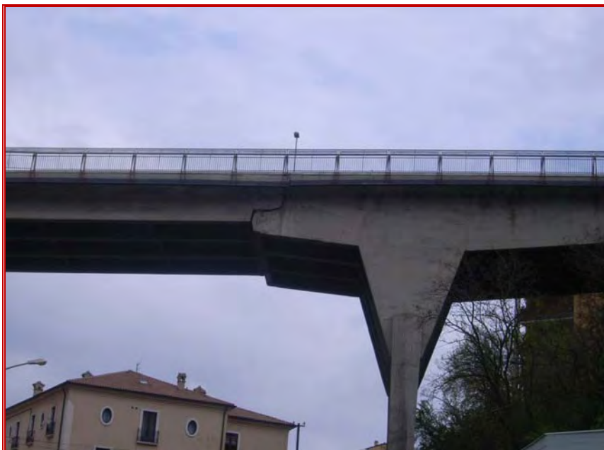
Figure 50: View of propped cantilever bridge with displacement at connection.
