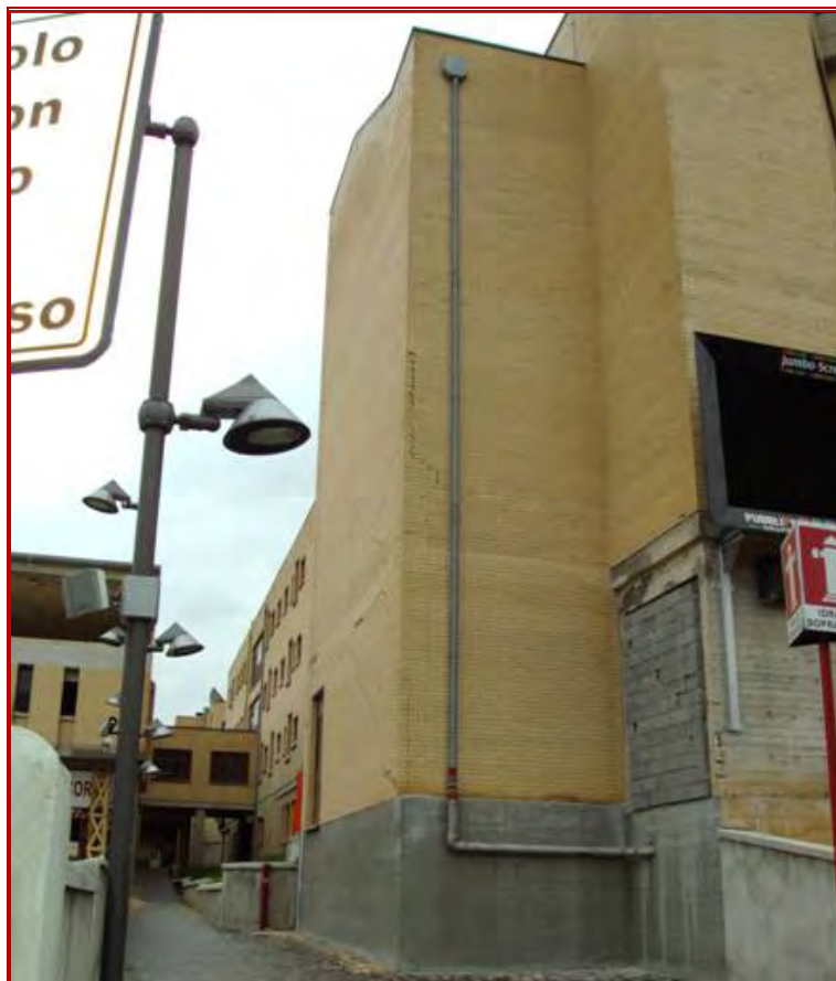
Figure 44. Shear cracks on the ground and first floors on one of the Northern hospital buildings. The concrete block infill wall on the right-hand-side of the photo was displaced from its axis about 3-5 cm.
