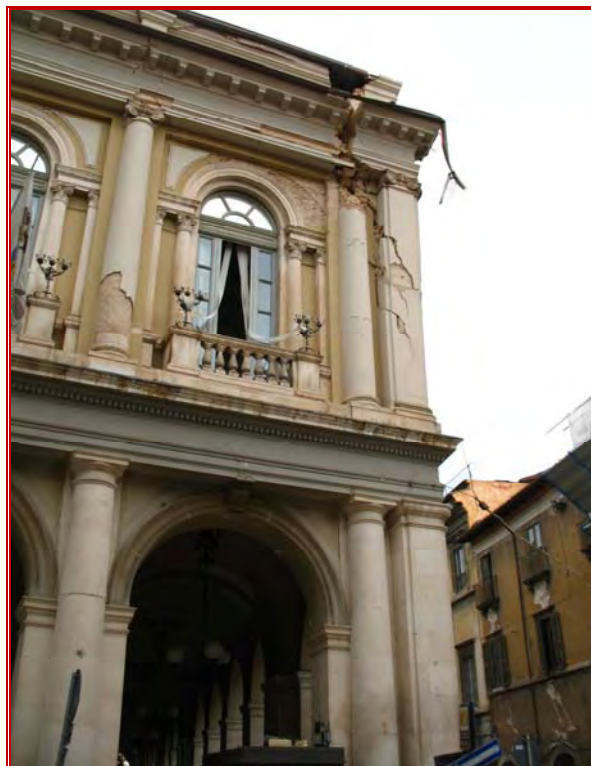
Figure 37: Damage to corner of government building in L'Aquila
