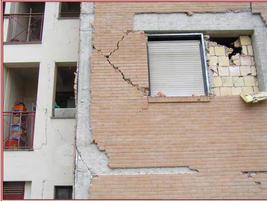
Figure 12: Detail of the 5 storey residential block at the top of the hill at Pettino, showing shear cracks in beam-column connection and infill panel failure.
