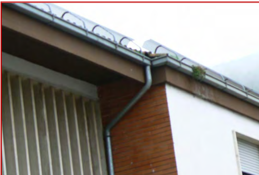
Figure 48: Detail of a school in Lucoli where brackets and wire mesh had been placed to prevent falling of roof tiles.
