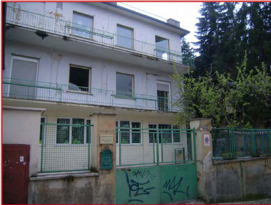
Figure 47: Elementary school in Aquila. RC frame building with infill, which sustained slight damage.
