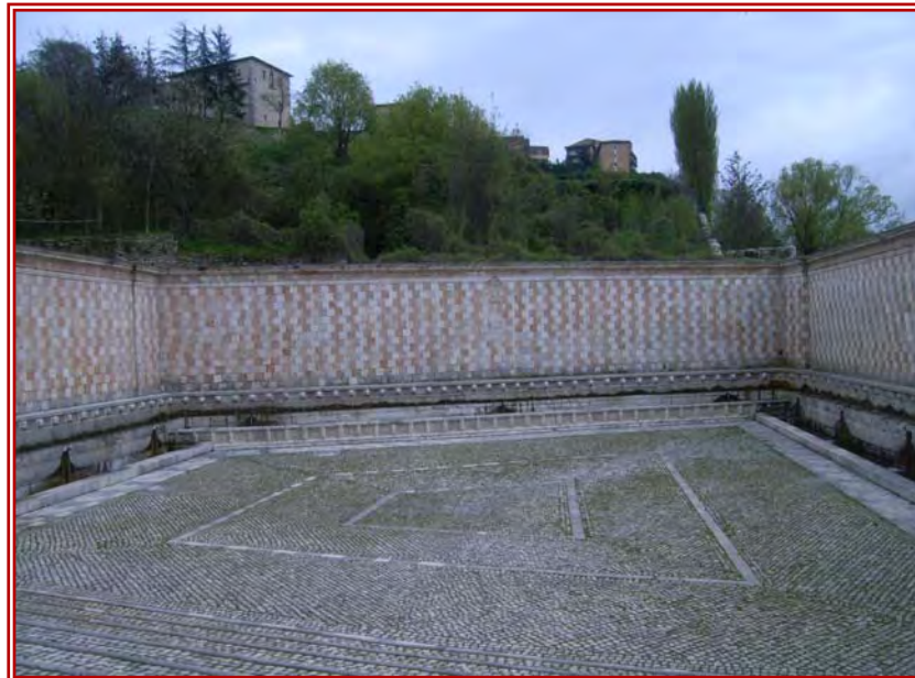
Figure 9: The Fontana della Riviera after the 6 th April 2009 earthquake
