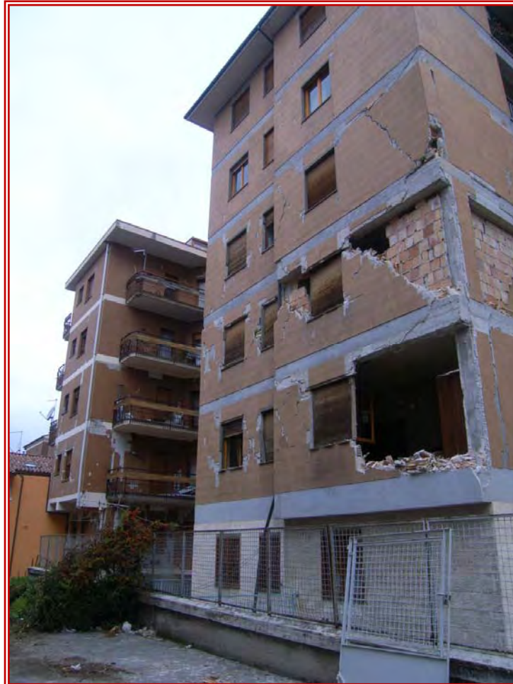
Figure 25: RC frame in Aquila Centre with severe damage to infill but intact structural frame.
