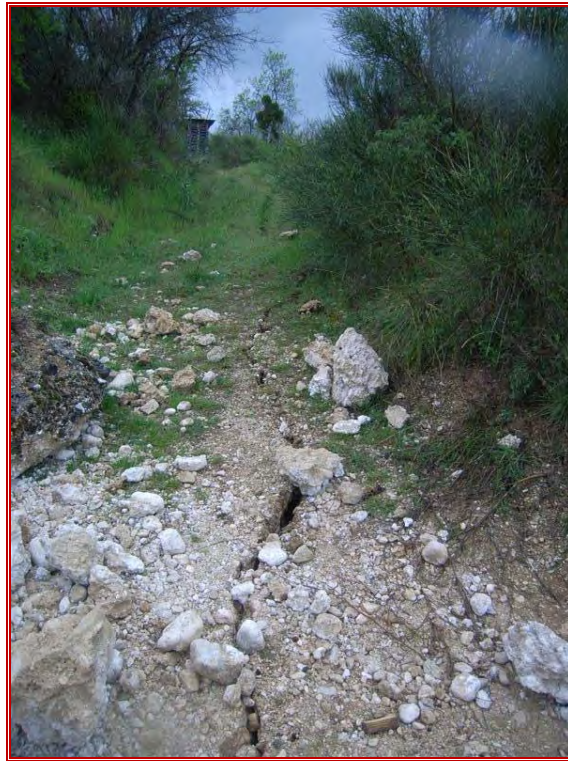
Figure 55: Tension crack in the hillside above Paganica Town
