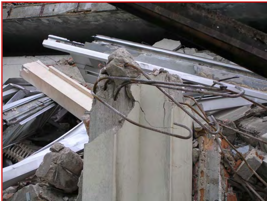
Figure 30: Detail of failed column from Hotel degli Abruzzi in Aquila
