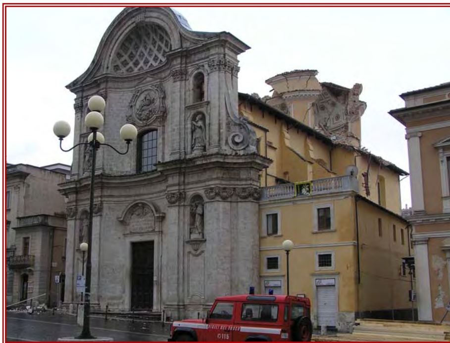
Figure 8: Church of Santa Maria del Suffragio, which dome was damaged during the April 6, 2009 event.
