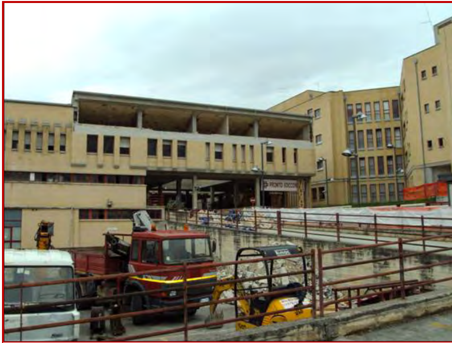
Figure 43: Northern blocks of L'Aquila hospital. Note that the infill walls on the top floor of the entrance collapsed.
