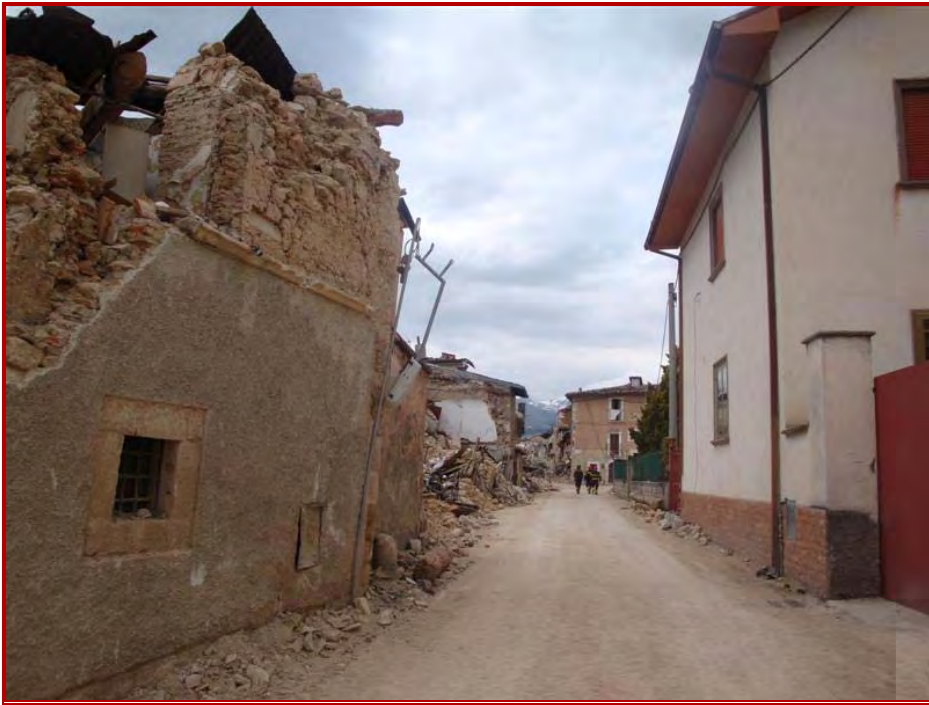
Figure 16: View of partially collapsed masonry building (left) and negligibly damaged reinforced concrete building (right).
