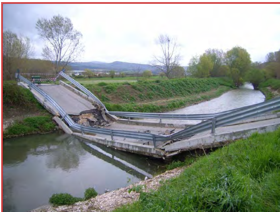
Figure 51: Failed minor road bridge at Fossa
