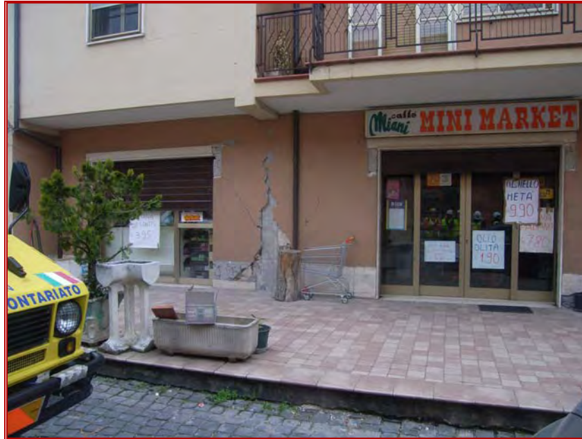
Figure 19: Reinforced Concrete frame structure with damage to infill panel
