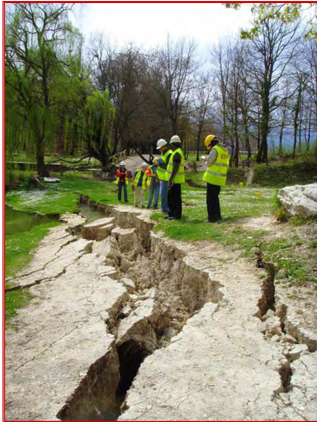
Figure 59: Slumping in fill around the edges of Lago Sinizzo.
