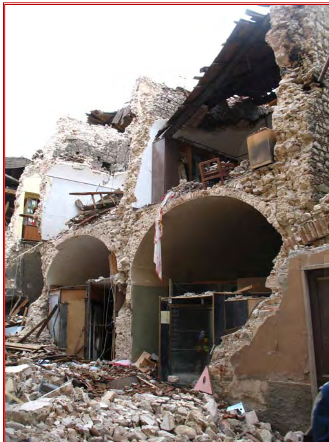
Figure 34: Building typologies - a major collapse opposite University Building in L'Aquila showing the typical masonry wall construction and vaulted floor construction.
