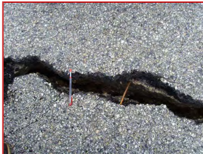
Figure 54: Tension crack at Paganica
