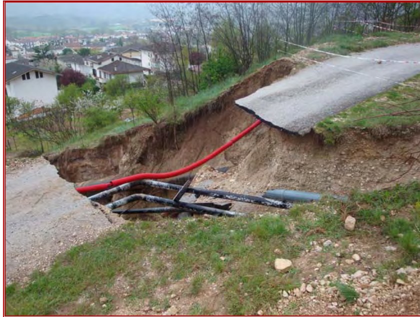
Figure 52: Failed water main at Paganica
