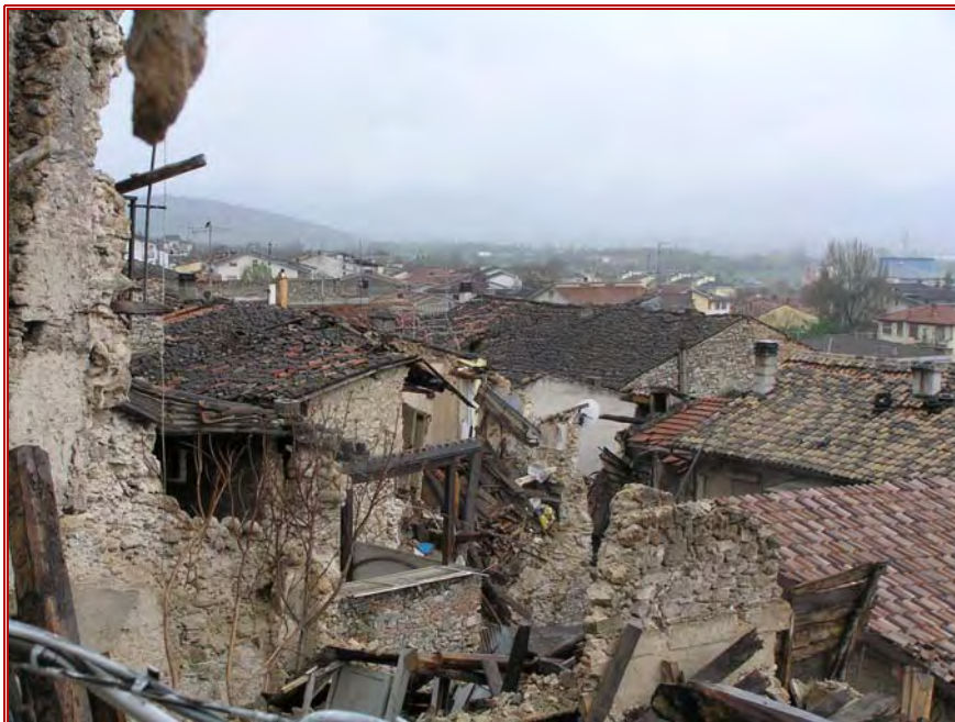
Figure 23: Panoramic view of damaged masonry houses in Paganica
