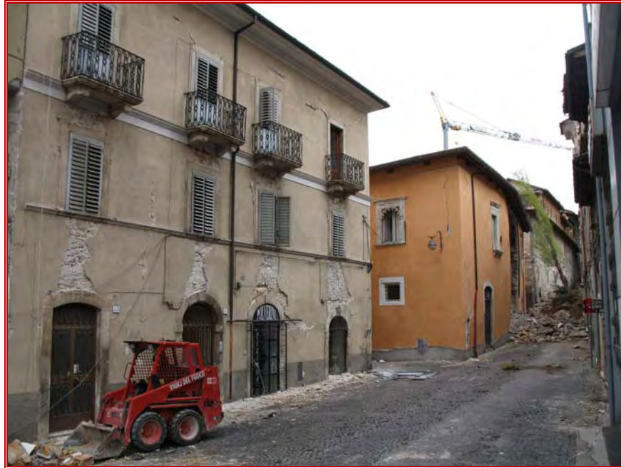
Figure 38: Typical minor to moderate damage to masonry buildings in L'Aquila
