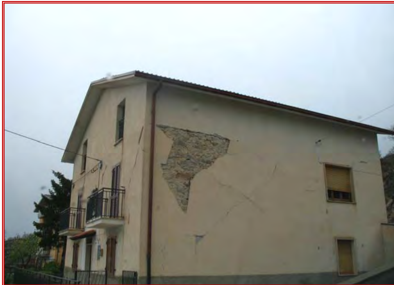
Figure 35: Building typologies - building in Poggio di Roio with concrete slab roof. Falling render shows how the presence of concrete roof and slabs exists with stone masonry wall loadbearing walls
