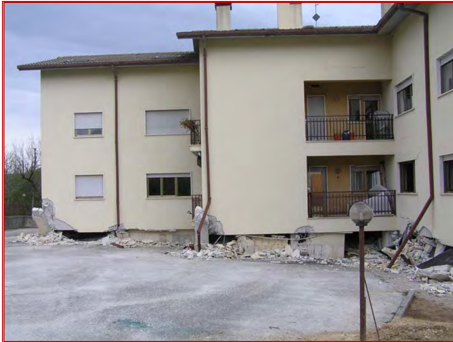
Figure 26: Three storey RC frame with soft-storey failure in Pettino.
