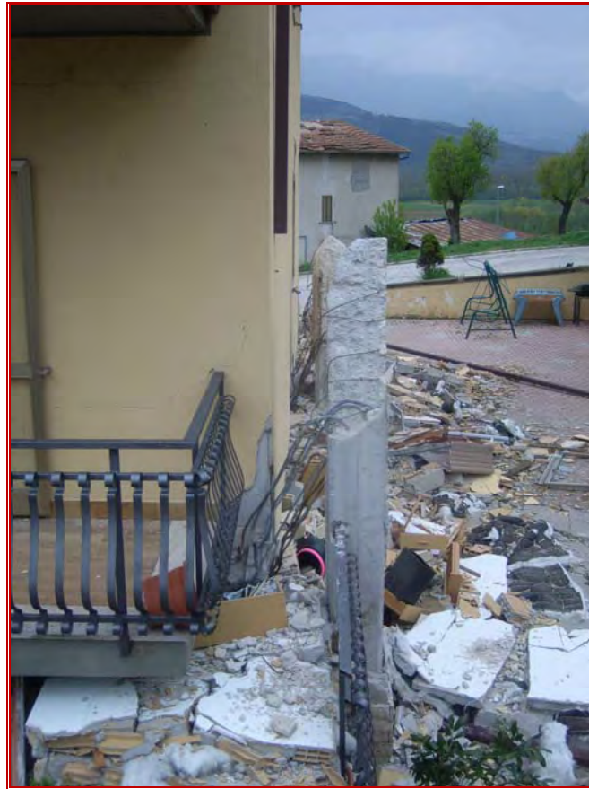
Figure 28: Detail of soft-storey collapse of RC frame in San Gregorio
