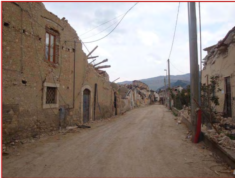
Figure 13: View to south down Onna main road showing very heavy damage (Grade 4) and destruction (Grade 5) of typical masonry buildings.
