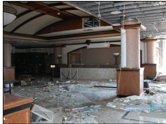
(b) Interior Damage
