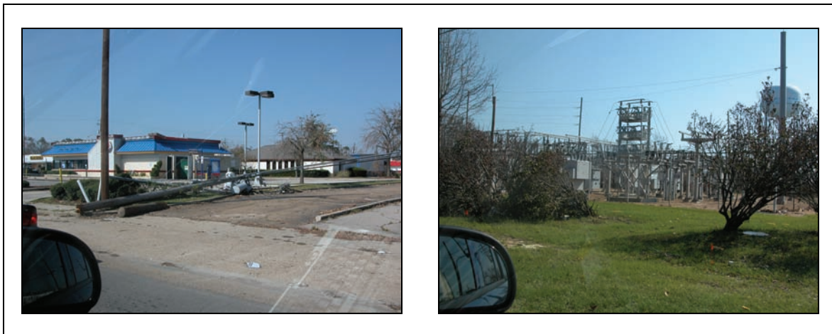
Figure 5-1. Downed power pole with poletop transformer; exposed substation equipment in Biloxi, MS, replaced by October 7.
