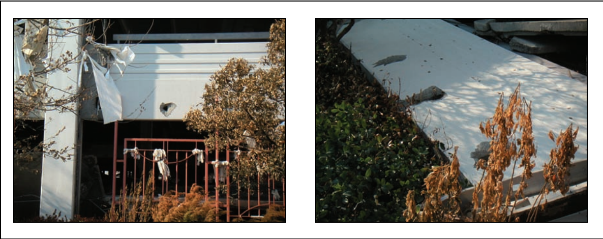
Figure 4-6. Evidence of horizontal pounding by waves. Deck-beam shear key appears to have punched holes in the spandrel beam.
