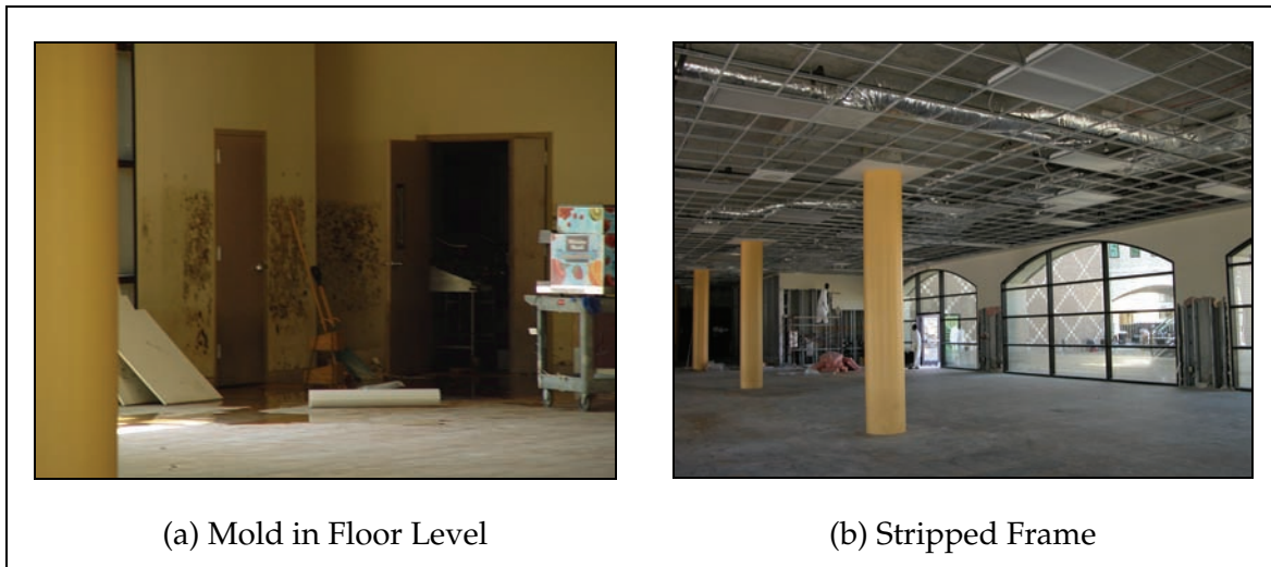
Figure 3-21. Flood damage to new student center in university near New Orleans.
