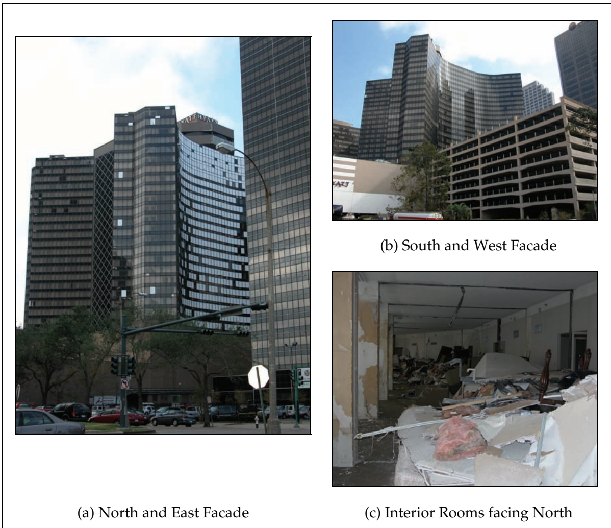
Figure 3-2. The Hyatt Regency Hotel in the New Orleans Business District had extensive window damage on the north facade (a) and limited damage on other sides (b). Broken windows allowed wind-driven rain and debris into the building causing additional interior damage (c).
