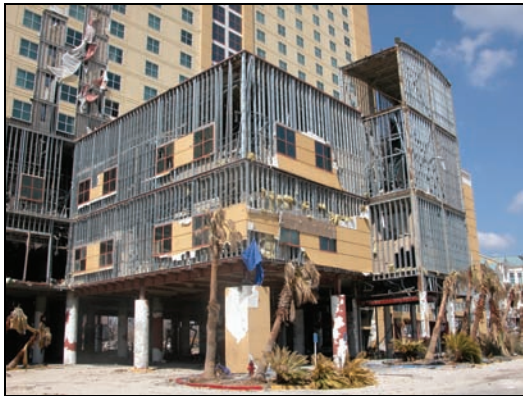
(a) Exterior Damage
