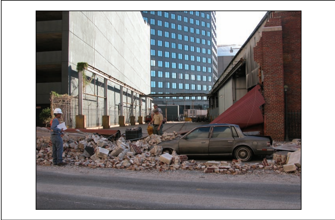
Figure 4-3. Collapsed unreinforced masonry wall.
