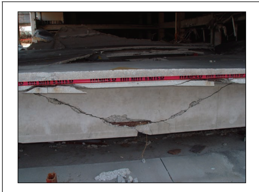
Figure 4-14. Spalling of concrete at the bottom fiber of deck beams.
