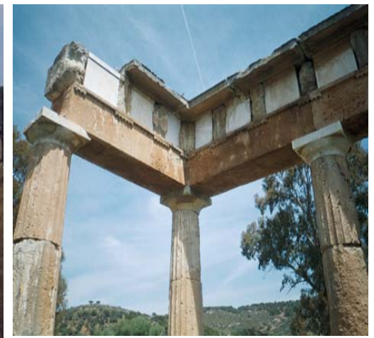
Brauron - Birds nestling on the damaged roof of the stoa (field visit of 3/06/2007)
