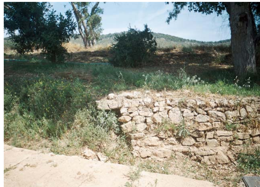
Erosion of the protective wall , NE corner (field visit of 3/06/2007)
