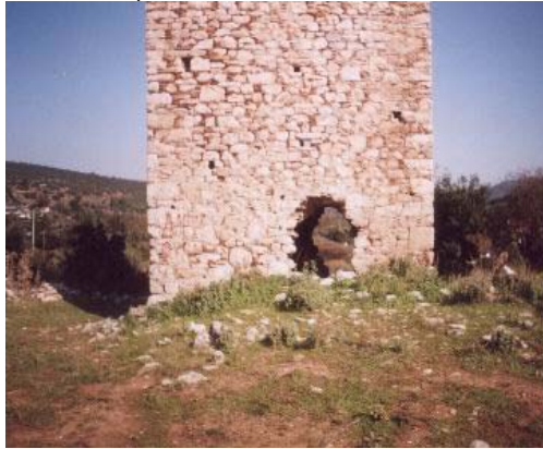
Oinoe Tower, NW view - fire danger from garbage & vegetation (field visit of 8/11/2006)
