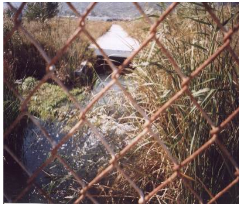
Drainage pipeline within the installations of ex-American Base at Nea Makri, 8/11/2006)
