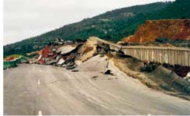
Fig.37.6. Malakasa landslide, February 1995. Damages on the new highway from Athens to Thessaloniki. The landslide manifested in the tectonized and weathered zone of schists covered by debris
