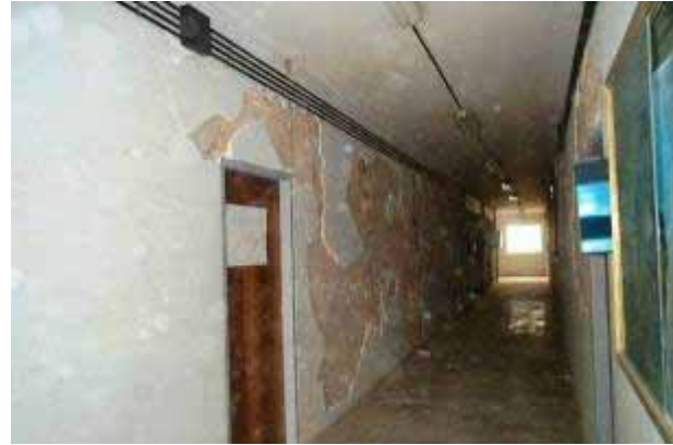
Interior corridor, damage to walls
