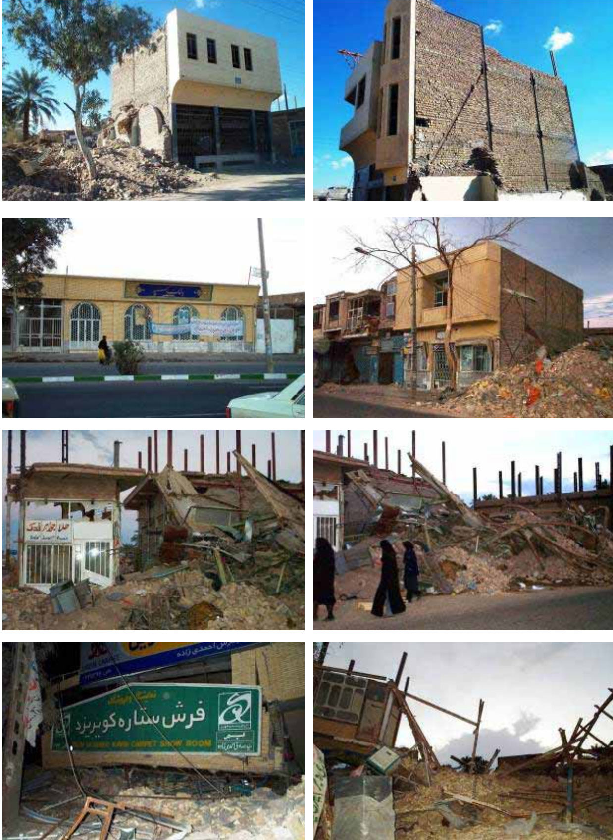
Figure 45: Performance of steel structures under Bam earthquake. Upper two rows: Braced frame structures that resisted major damage and collapse. Lower two rows: Unbraced and poorly constructed steel structures in jewellery market of Bam and surrounding area that suffered complete collapse.
