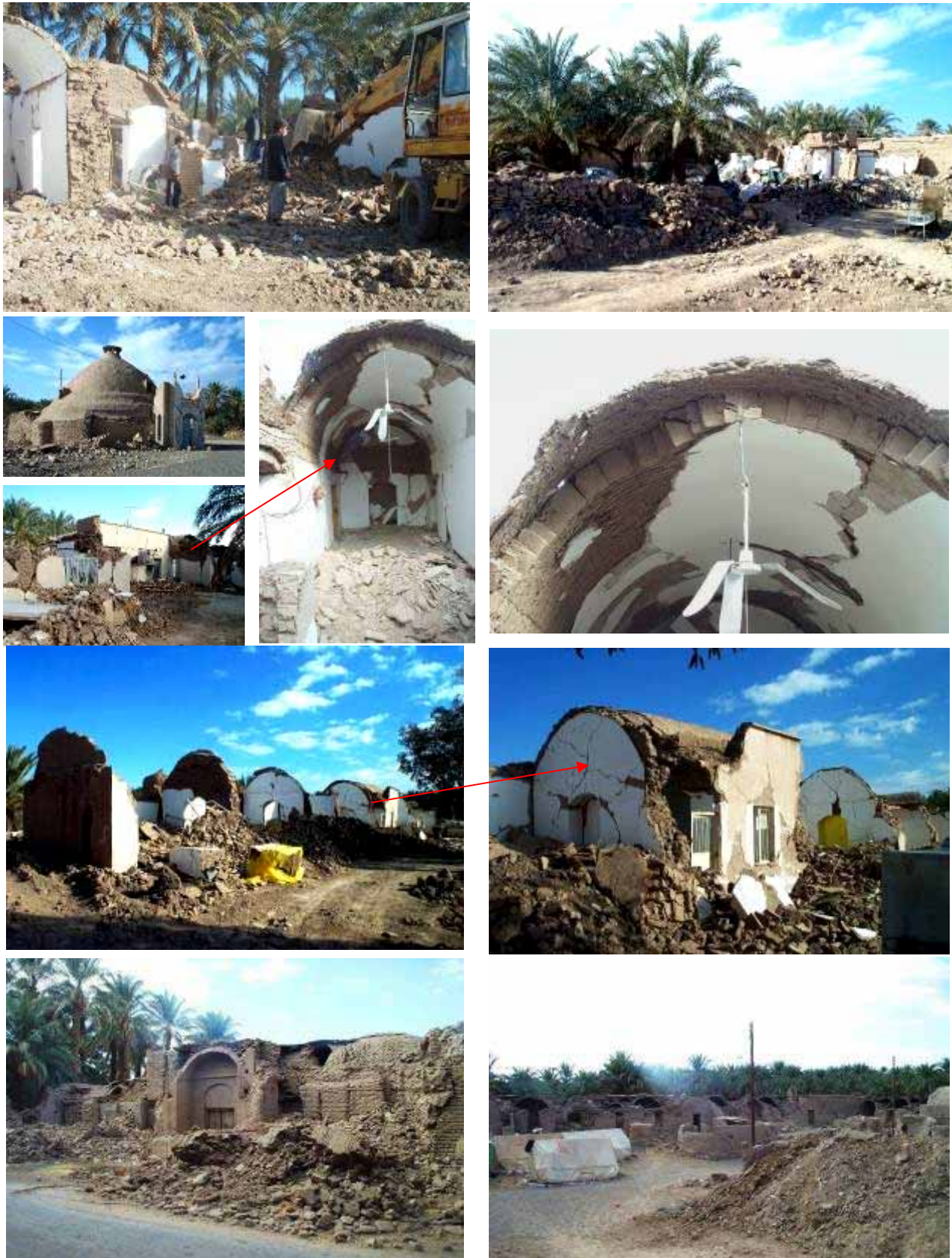
Figure 23: Damage to mud-brick building in villages-(Rows 1 to 3: Esfikan Village, North of the Bam) 1 st row: total collapse, 2 nd row: Traditional sport facility (Zoor-Khaneh) with cracked domed roof, a collapsed mud-brick house and details of barrel vaulted roof, 3 rd row a part of boys Guidance School, 4 th row: damage in Nartij Village, northwest of Bam
