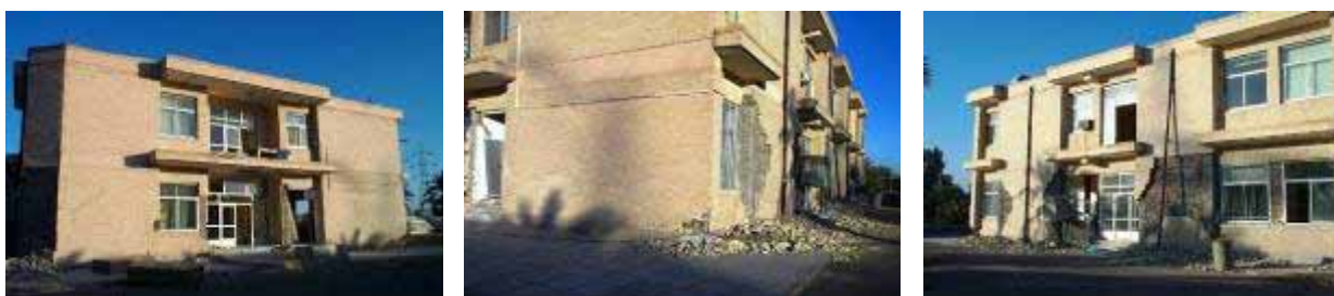
Damage to the building viewed from outside
