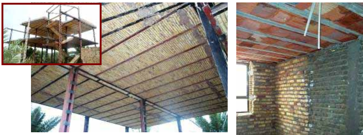
Figure 27: Jack-arch flooring system in a steel frame structure (left) which is very common throughout Iran, and hollow brick-RC joist floor system in a masonry building the other common alternative (right). Pictures from Bam.
