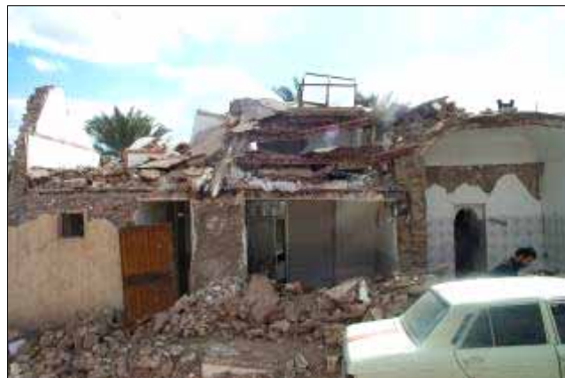
Figure 26: A combination of traditional and modern masonry construction materials and methods. Mud-brick walls (right) and fired brick walls (middle and left) has been extended in second floor by fired brick walls and vaulted roof (left) and jack-arch roof (middle). Second floor completely collapsed.
