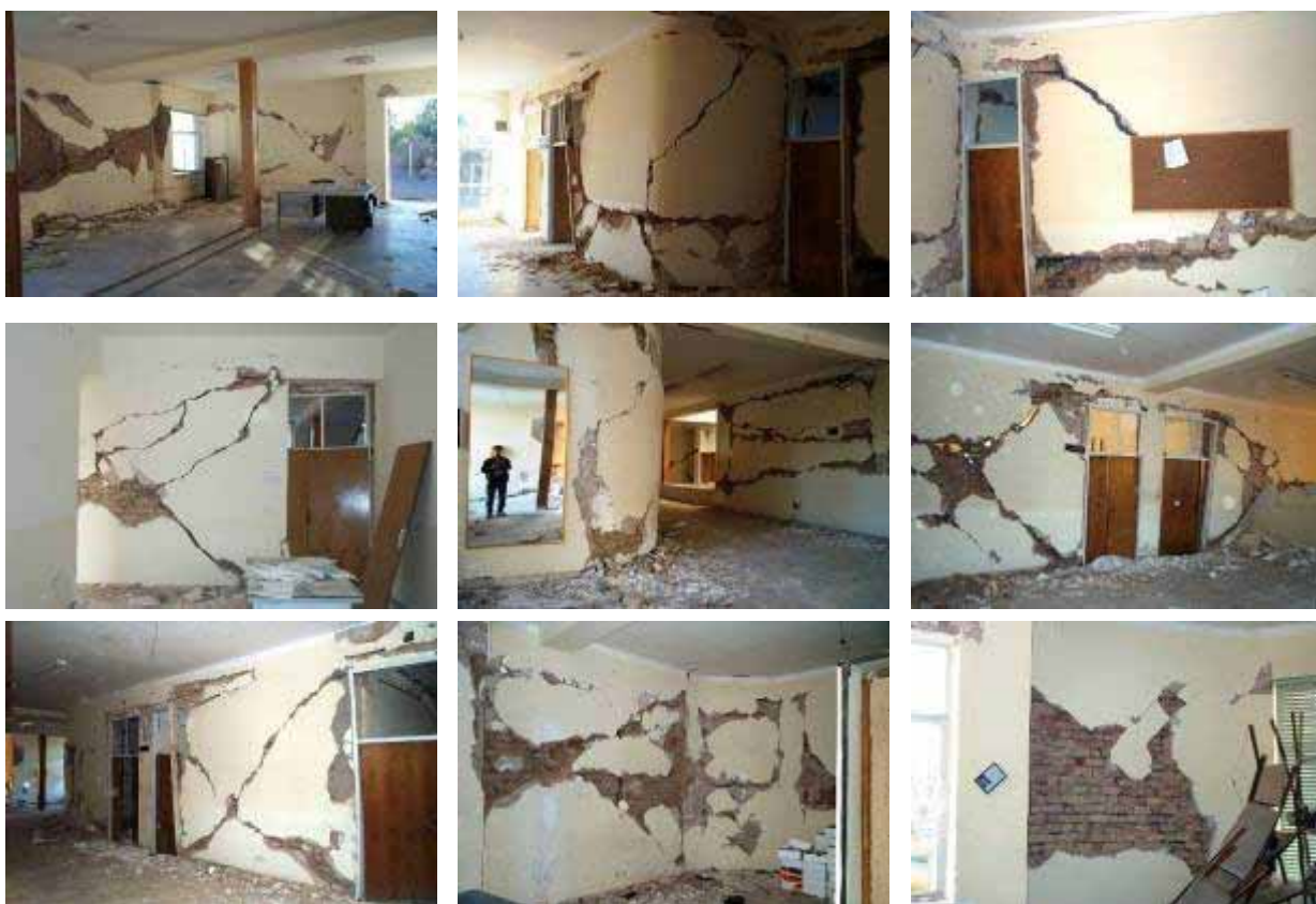
Damage observed from inside the building at the first floor level
