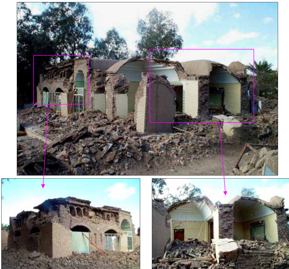
Complex vaulted roof construction with flat finishing, resulting in a heavy roof
