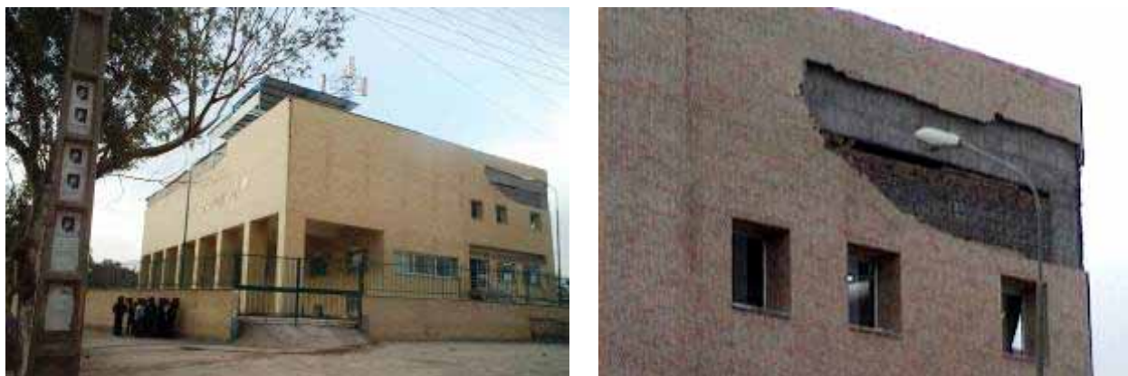
Figure 47: Bam’s Emamat Telecommunication Complex in Zied square. RC frame structure with damage to facade at various locations. Otherwise the structure appeared to be intact. (interior of the building was not visited).
