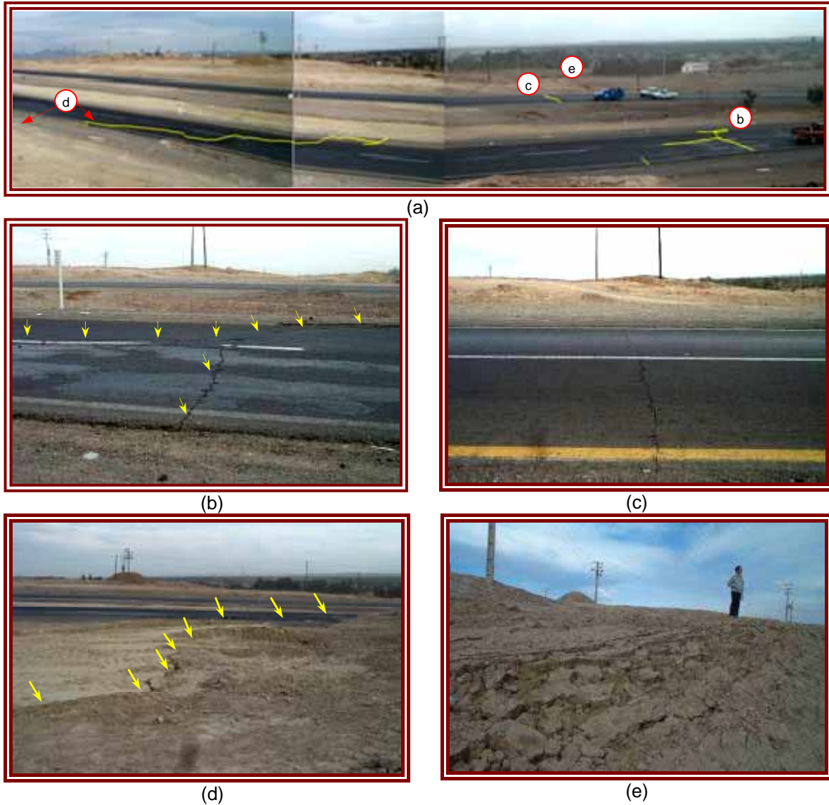
Figure 6: Ground movements along the Bam fault on the Bam-Baravat road and nearby ground (a) panoramic view on Bam-Baravat road from south with cracked areas highlighted (b), (c) Close up view of cracks in south and north band of the road (d) Cracking in the ground on the south side of the road (e) a shattered zone of fissures on the north side (Yellow lines and arrows show the location of cracks)
