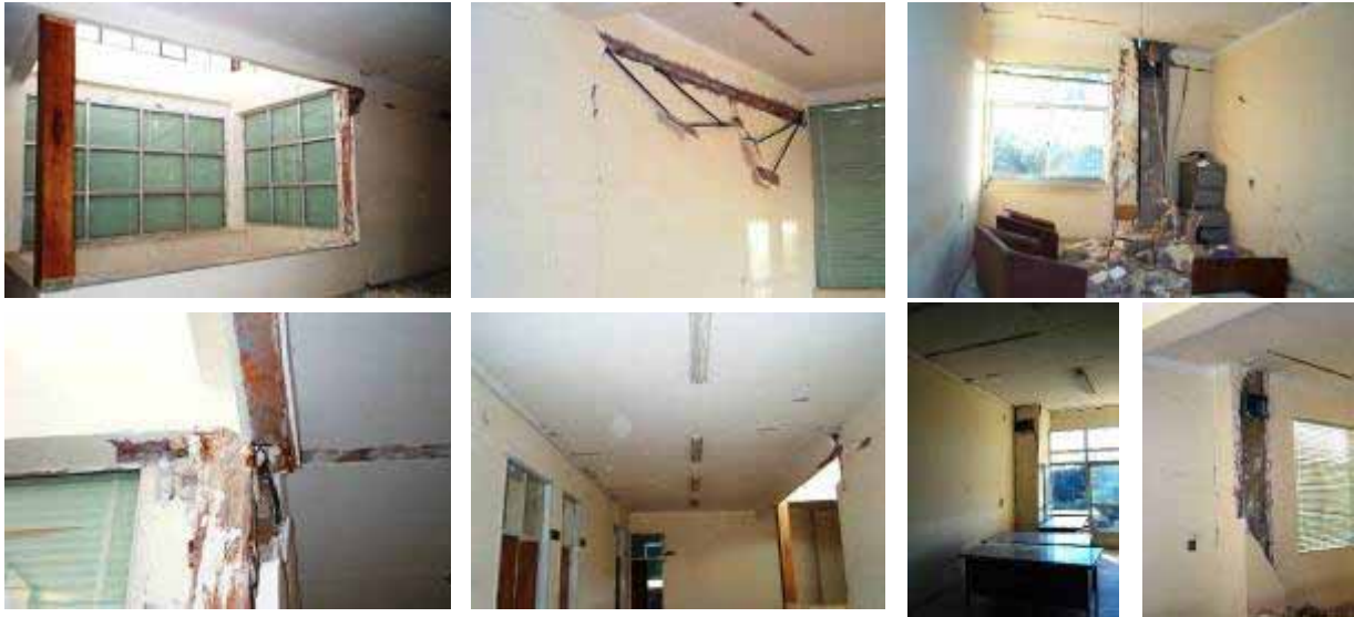
Damage in second floor
