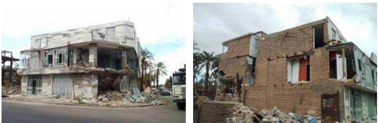
Figure 40: An example of inferior construction of a steel structure located in the neighbourhood of Imam hospital in Bam. Note the irrational bracing configuration at the side of the building.
