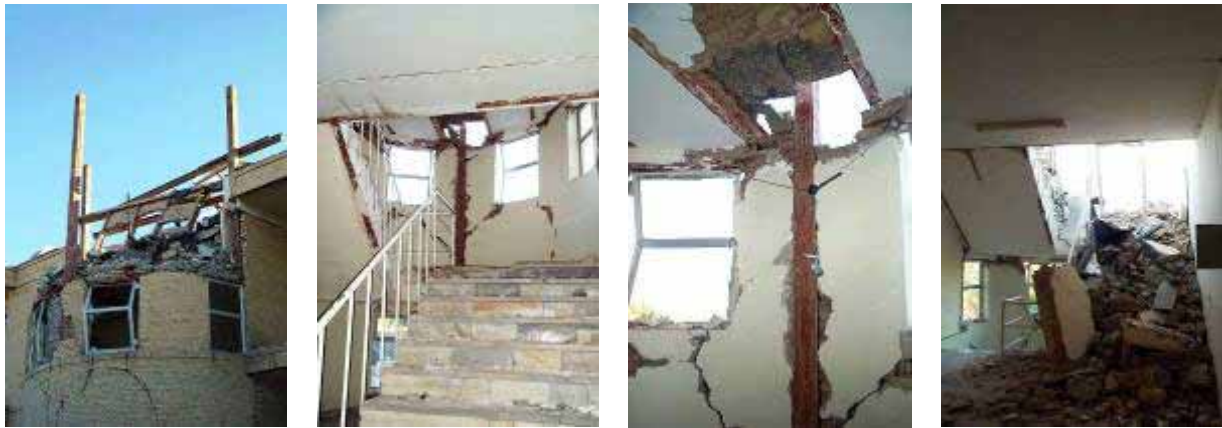
Damage to staircase viewed from outside and inside the building
