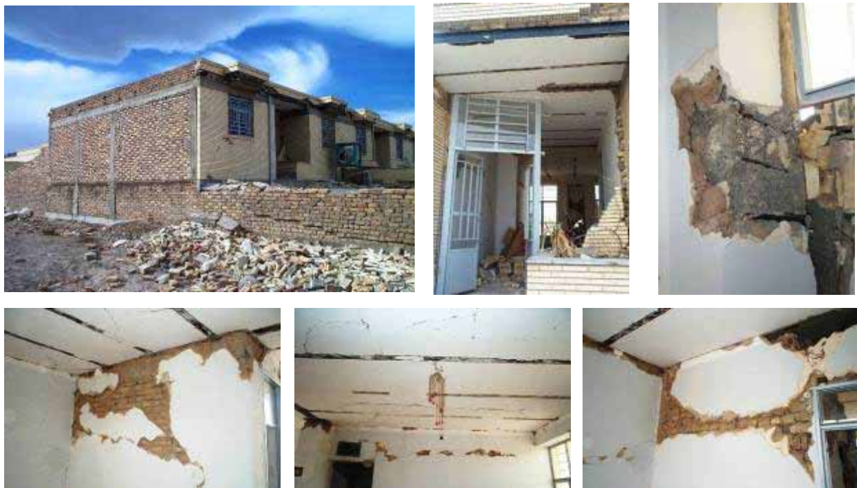
Figure 33: Bonyad Maskan houses for teachers in Baravat. The buildings have vertical and horizontal ties. Some of the vertical ties were observed not to start from foundation level (top left). Walls surrounding the courtyard collapsed. Although the structure did not collapse it suffered structural and non-structural damage in the form of large cracks in the walls and the roof magnified by the poor quality of building materials and construction.
