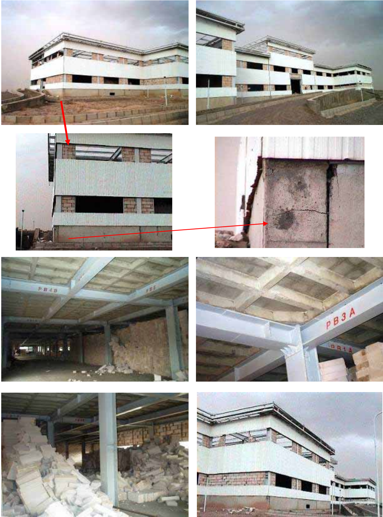
Figure 50: A new hospital under construction at the time of the Bam earthquake, about 1.5km to the west of the Bam fault line on the Bam-Baravat road. The structural system is steel frame with precast two way spanning ribbed concrete floors. Some concrete blocks of infill walls, mostly in the top floor, collapsed but no structural damage was observed.
