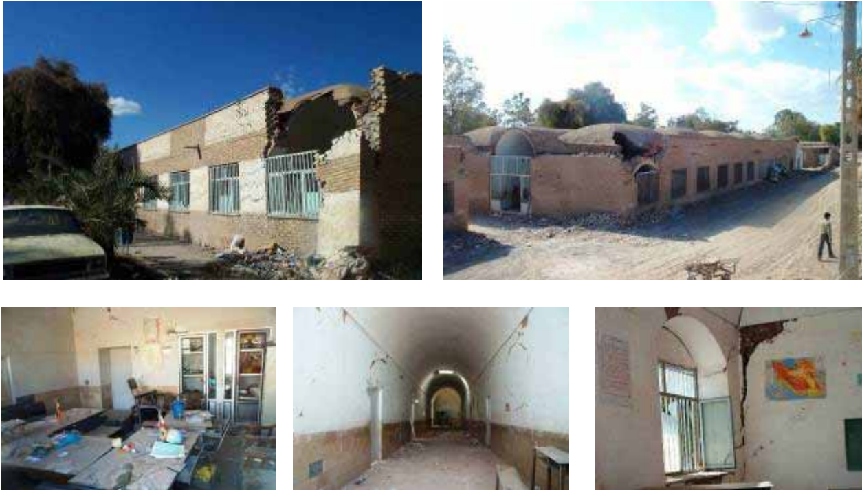
Figure 32: Adab girls' school in Bam city centre. A typical example of masonry buildings with fire brick vaulted roofs. This building has a double spanned vaulted roof at two sides and a barrel vaulted roof in the middle. Both roof corners and most of the parapet on the end wall collapsed, but elsewhere the building survived without collapse. Also, damage to walls and roofs from the inside of the building, mainly in form of minor to large cracks, were observed.
