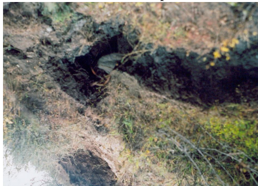
Cracks on the slope at Jula village, Uri
