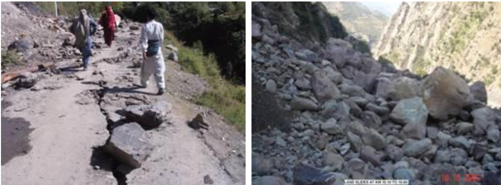
Damaged and blocked Uri-Kaman Post-Muzzaffarabad Road sections
