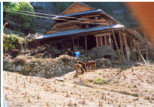
Upslope tilting of the structure at Kamalkot
