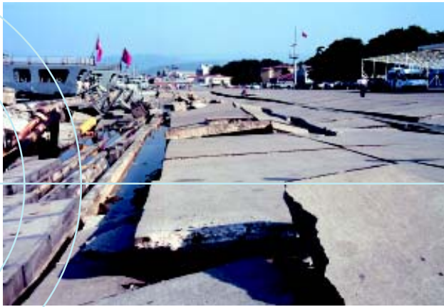
Damage due to faulting and lateral spreading at the main pier and seawall of the Gölcük Naval Base.
