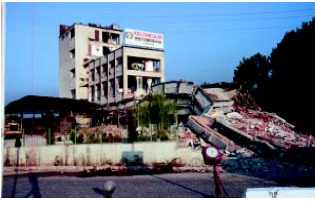
Reinforced concrete industrial building at Gölcük. The front third of the building has collapsed completely. The middle section has two floors collapsed.
