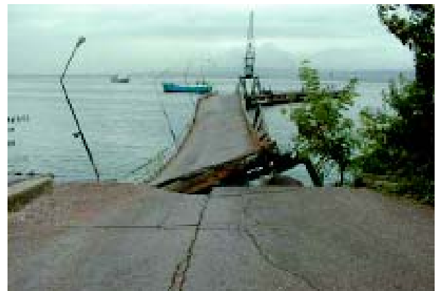
Damage to a bridge to the pier at the SEKA Paper Mill in Izmit.
