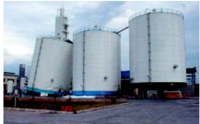
Identical liquid oxygen and nitrogen tanks at Habas facility in Izmit. Reinforced concrete supports collapsed on full tanks left and center, but not on 1/4 full tank on right.
