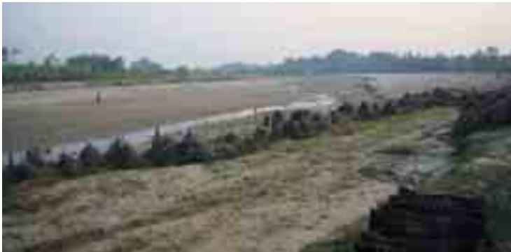
Figure 19: Embankment made out of bamboo constructed by a local NGO using local knowledge and local material. Phoolparasi VDC, Sarlahi District
