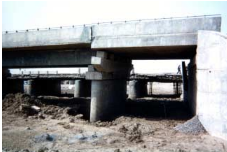
Figure 2.46. Damage to RC highway bridge under construction approximately 35 km east of the USGS epicenter. Photo courtesy of Charles Menun.
