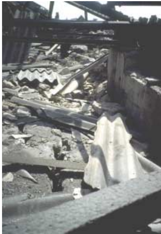
Figure 2.36. Lateral spreading due to liquefaction initiated collapse. Note the wide fissure inside the building footprint. Photo courtesy of Charles Menun.
