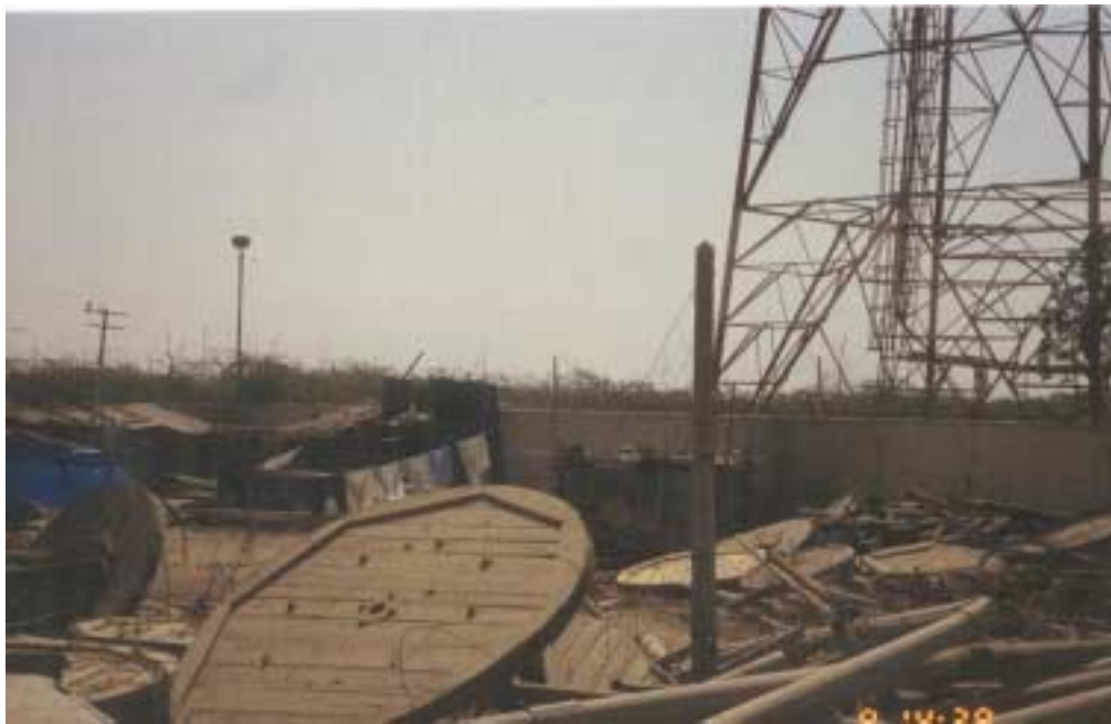
Figure 3.3. Destruction outside the Communications Center for Kachchh District, Gandhidham, March 2, 2001. Tower remained standing.
