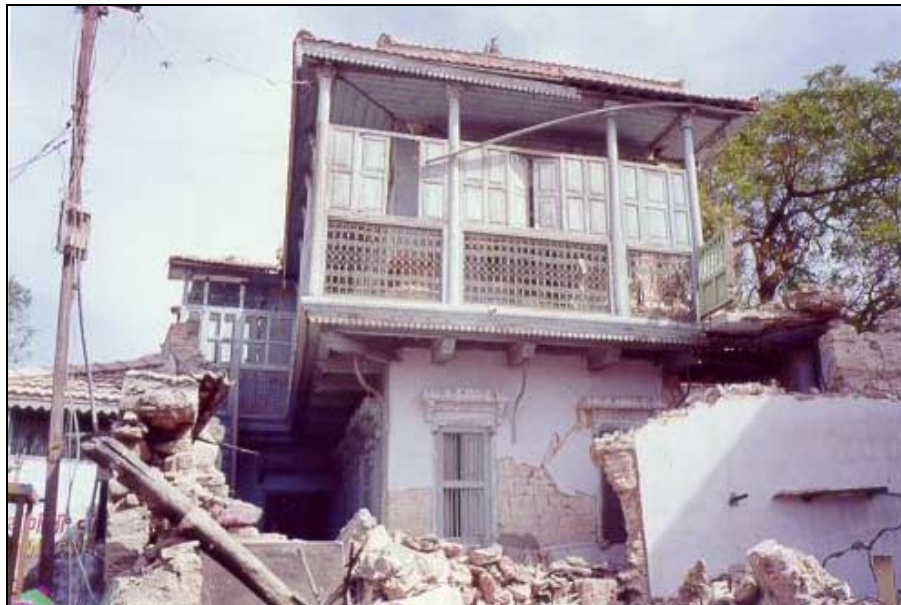
Figure 4.9. A damaged but still standing house of wooden construction, Anjar.
