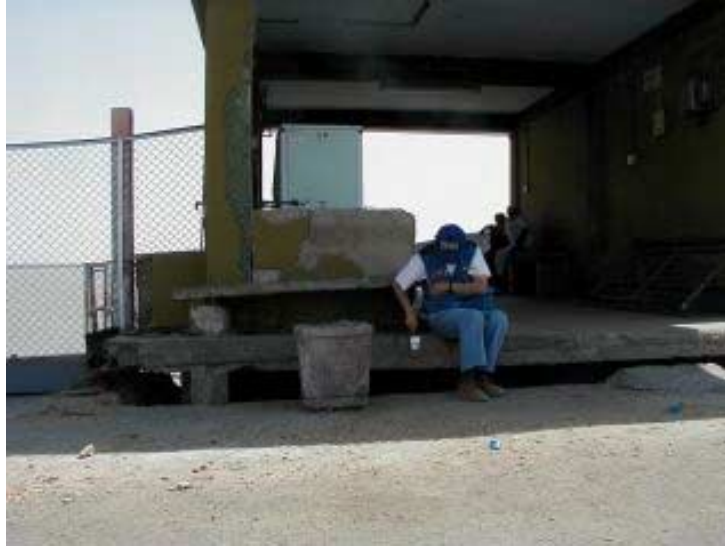
Figure 2.37. Subsidence of ground relative to pile-supported structure. Photo courtesy of Tetsu Masuda.
