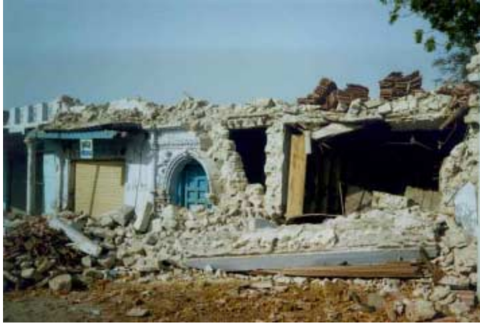
Figure 2.13. Damage to cutstone and lime mortar masonry building in old Bhuj. Photo courtesy of Ahmad Naderzadeh.
