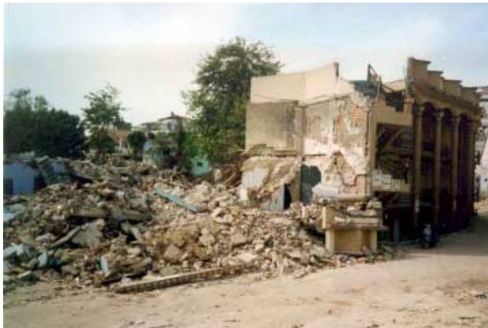
Figure 2.8. Collapse of a stone masonry house in Anjar. Photo courtesy of Ahmad Naderzadeh.
