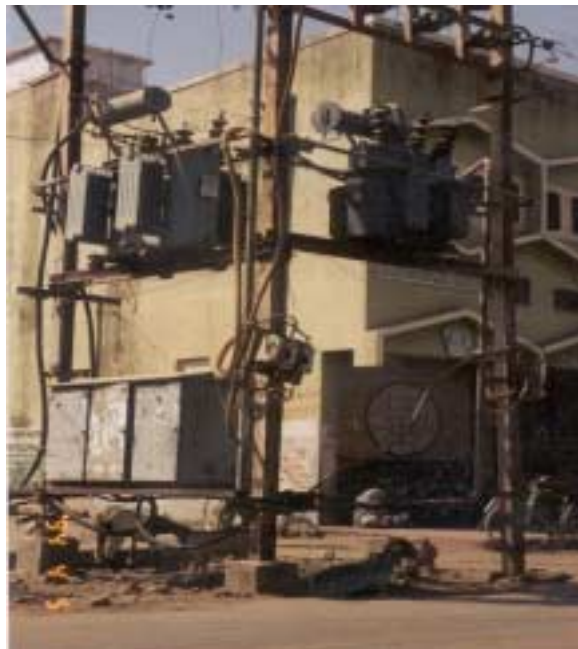
Figure 3.7. Electrical transmission station in Limdi, February 27, 2001.
