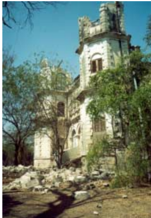
Figure 2.14. Damage to the tower and parapets of a palace in Limbdi. Photo courtesy of Svetlana Uranova.
