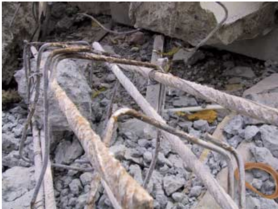
Figure 2.24. Damaged column from the Ayodhya apartment complex shown in Figure 2.19. Note the large column tie spacing and the use of 90° hooks. Photo courtesy of Weimin Dong.
