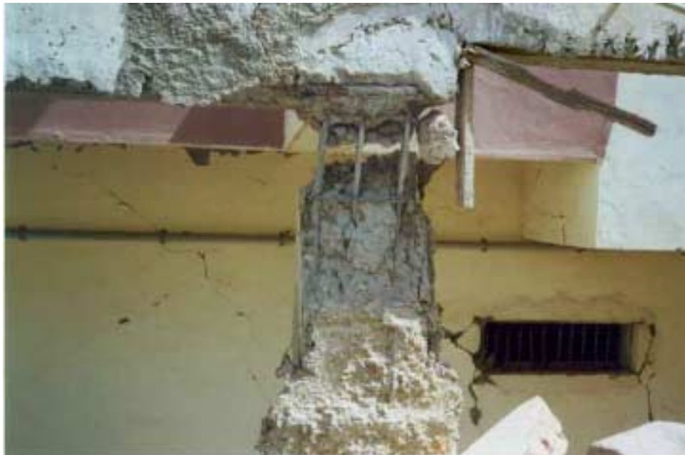
Figure 2.32. Poor quality concrete and lack of seismic detailing evident in beam column connection. Photo courtesy of Ahmad Naderzadeh.
