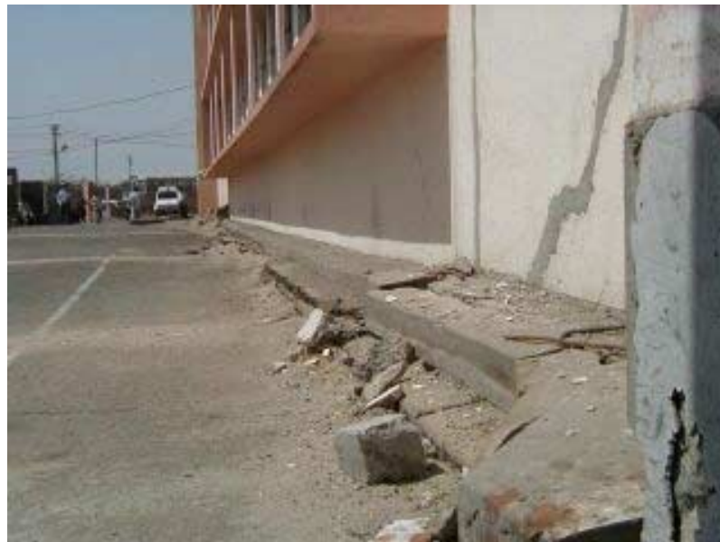
Figure 2.38. Subsidence of ground relative to pile-supported structure. Photo courtesy of Tetsu Masuda.
