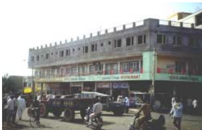
Figure 2.5. Buildings that performed well in Anjar were located only 2-3 blocks from location where the photos in Figure 2.4 were taken. Photos courtesy of Charles Menun.
