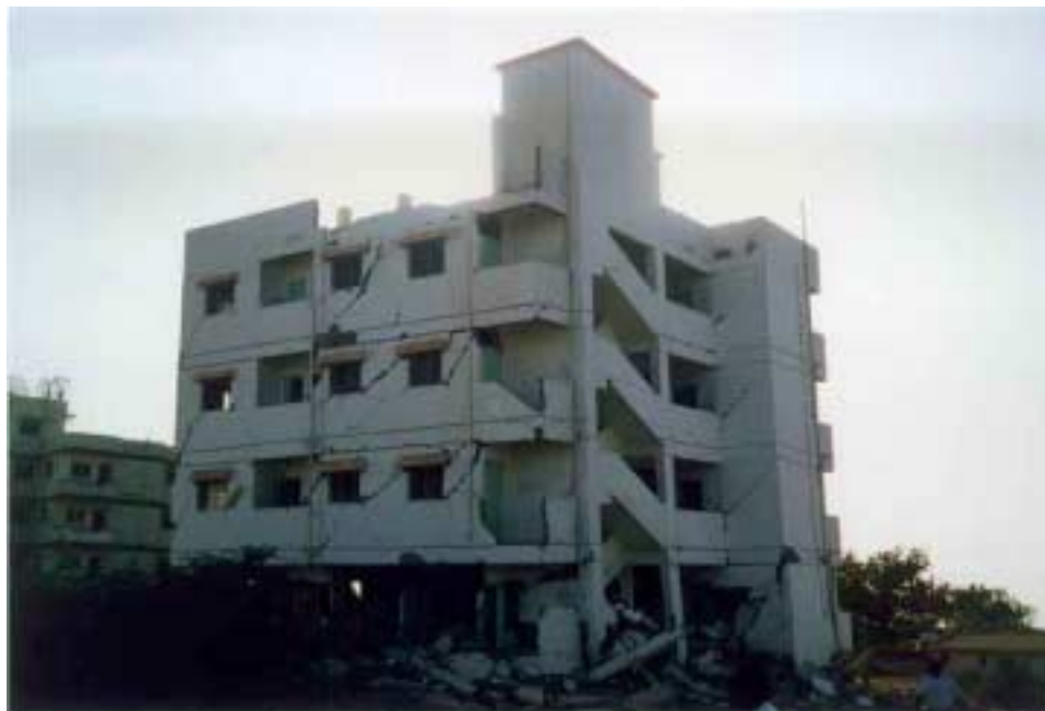
Figure 2.22. Different view of soft story collapse shown in Figure 21. Note the location of the water reservoir at the roof level relative to the floor plan. Photo courtesy of Ahmad Naderzadeh.
