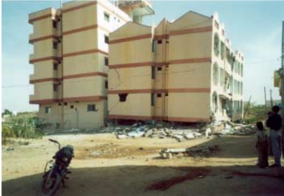
Figure 2.23. Komal Vihar Apartments, Bhuj. Collapsed building resulted from soft story effects. Photo courtesy of Svetlana Uranova.
