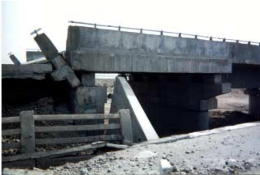
Figure 2.45. Damage to RC highway bridge under construction approximately 35 km east of the USGS epicenter. Photo courtesy of Charles Menun.
