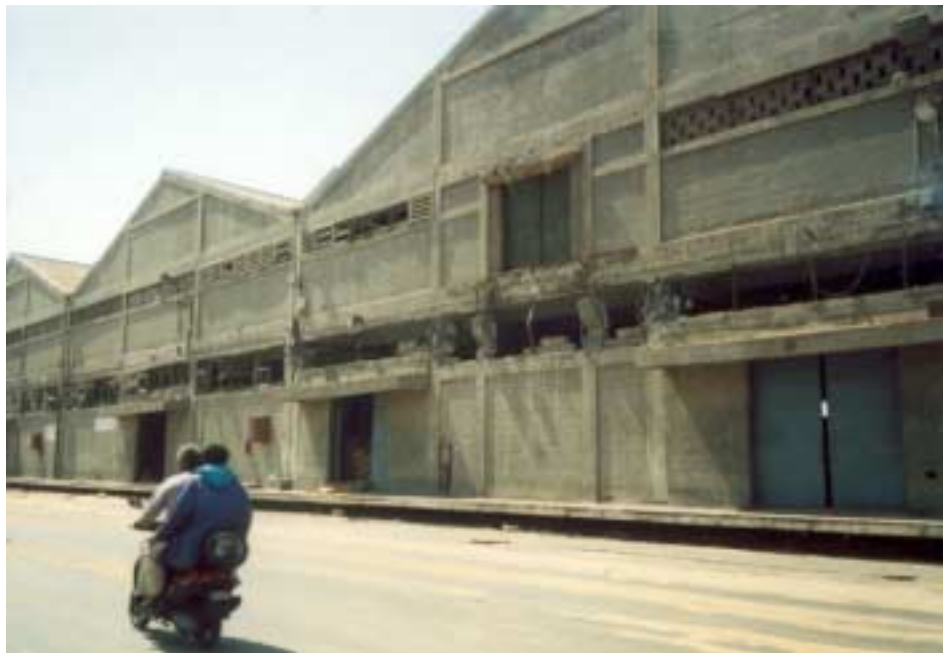
Figure 2.42. Damage to a warehouse at the port of Kandla due to short column effects. Photo courtesy of Svetlana Uranova.
