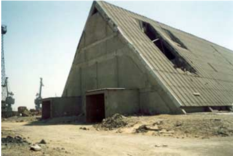
Figure 2.43. Partial collapse of roof of A-frame storage facility. Photo courtesy of Svetlana Uranova.
