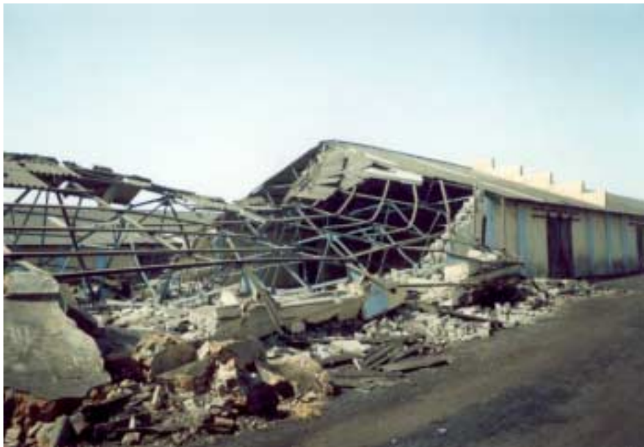
Figure 2.34. Collapse of a warehouse at the port of Navlakhi. Photo courtesy of Svetlana Uranova.
