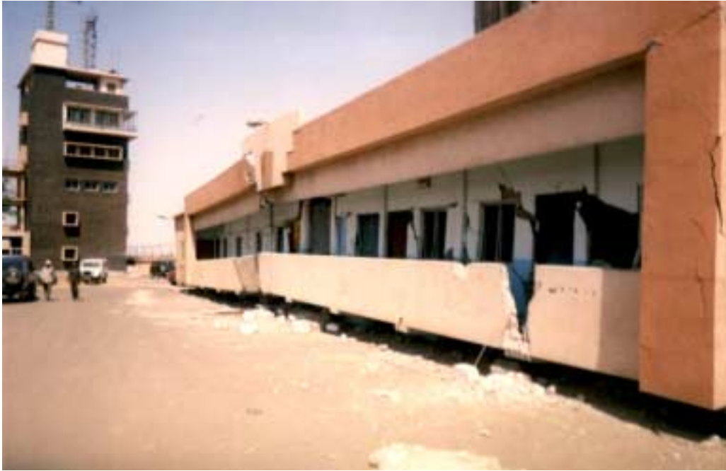
Figure 2.41. Soft story collapse of a two-story reinforced concrete building at the port of Kandla. Photo courtesy of Charles Menun.
