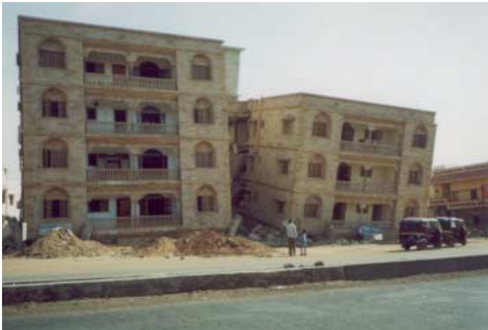
Figure 2.20. Taksila Apartments, Bhuj. Both 5-story buildings collapsed due to soft story effects. Photo courtesy of Svetlana Uranova.
