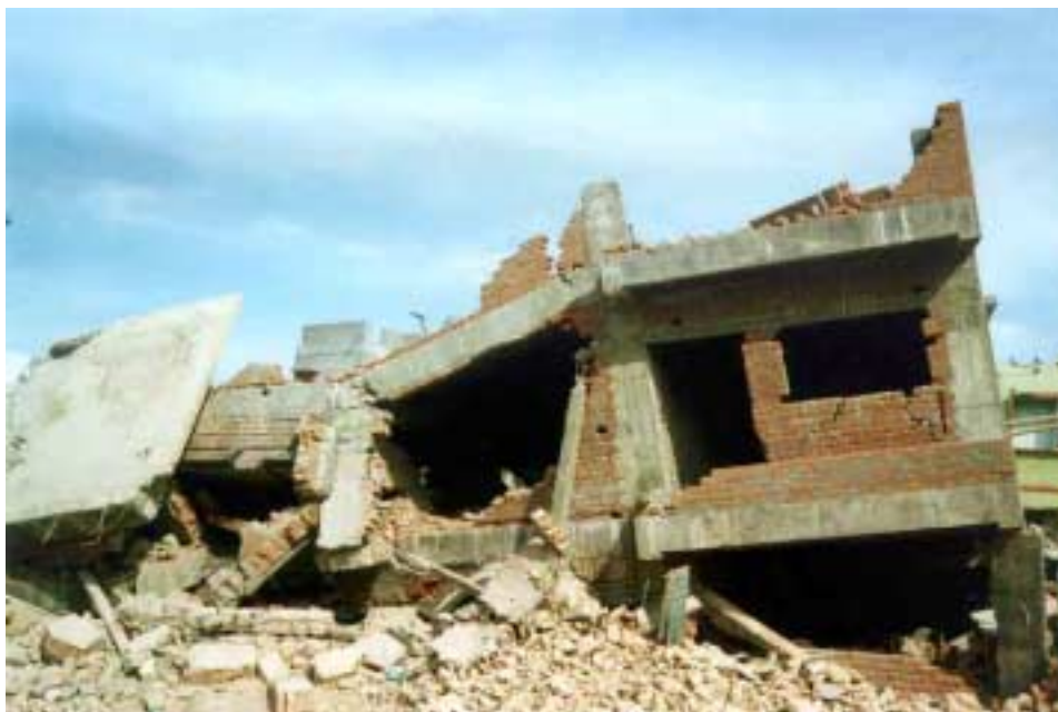
Figure 2.30. Damage caused by torsion due to unsymmetrical distribution of partition walls on the ground floor. Photo courtesy of Ahmad Naderzadeh.
