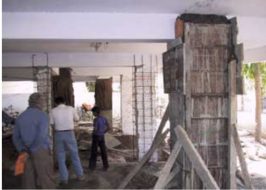
Figure 2.27. First floor of an apartment building in Ahmedabad being retrofitted without proper seismic design or details. Photo courtesy of Weimin Dong.
