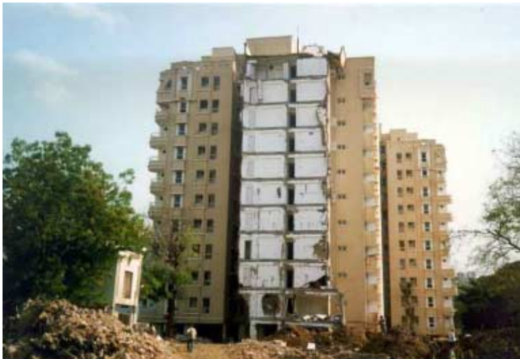
Figure 2.16. Shikhar Apartments, Ahmedabad. Building D (originally in foreground) collapsed due to soft story effects. Photo courtesy of Ahmad Naderzadeh.
