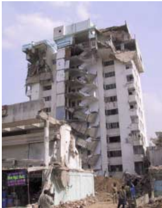
Figure 2.18. Manasi Apartments, Ahmedabad. 11-story building, in front of the building shown, collapsed due to soft story effects. Weight of swimming pool and reservoir at top of the collapsed building contributed to the severity of the damage. Photo courtesy of Weimin Dong.
