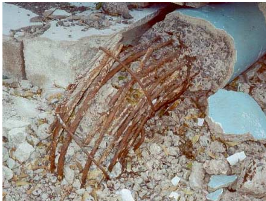
Figure 2.26. Reinforcement details of a column damaged in a soft story collapse. Note the congestion caused by lapping all of the longitudinal bars at one location. Also note the inadequate number of lateral ties over the splice length. Photo courtesy of Amod Dixit.
