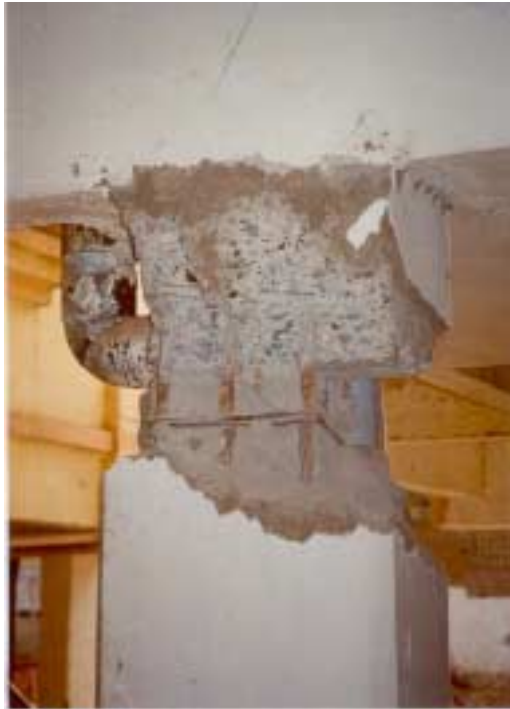
Figure 2.31. Ground floor column in Akshar Deep apartment complex, Ahmedabad. Photo courtesy of Amod Dixit.
