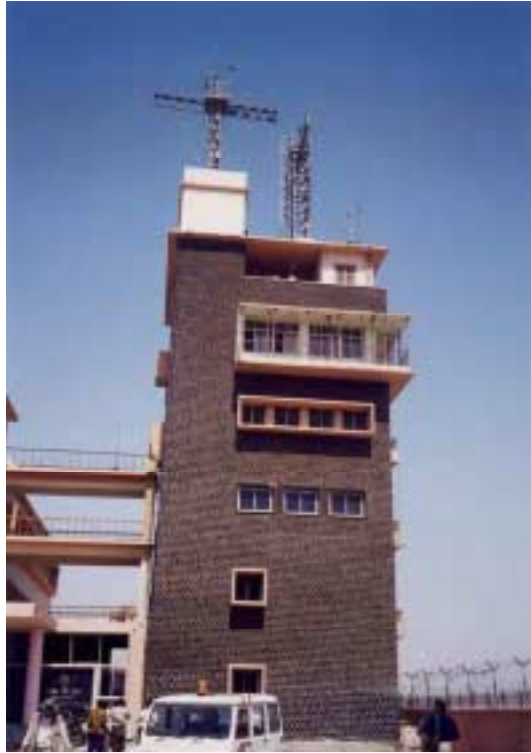
Figure 2.39. Port Authority Building, Kandla. Tilting of the control tower is due to settlement caused by liquefaction. Control tower is founded on piles. Photo courtesy of Ahmad Naderzadeh.
