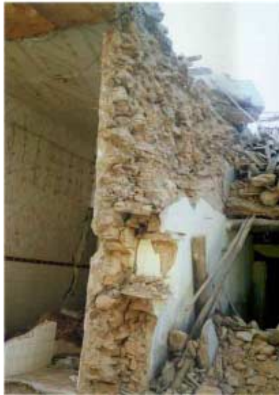
Figure 2.12. Damage to a rubble stone and mud mortar house in old Bhuj. Photo courtesy of Ahmad Naderzadeh.
