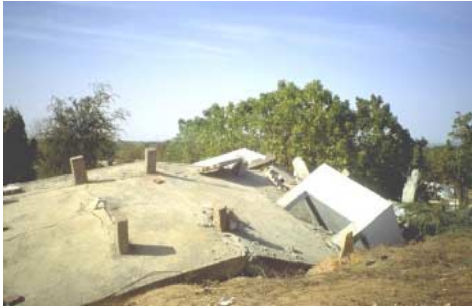
Figure 2.29. Roof level water reservoir perched on top of short columns. Location of the reservoir at a corner of the building amplified torsional motions and resulting loads. The photo shows the roof of a collapsed two-story RC building in Bhachau. Photo courtesy of Charles Menun.
