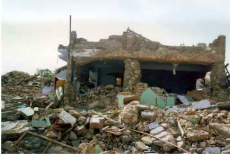
Figure 2.7. Damage to a stone masonry house in Anjar. Photo courtesy of Ahmad Naderzadeh.
