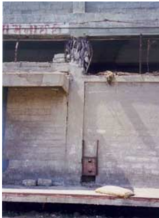
Figure 2.28. Damage due to short column effect in warehouse at the port of Kandla. Photo courtesy of Ahmad Naderzadeh.
