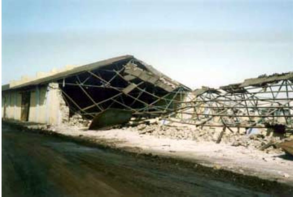
Figure 2.33. Collapse of a warehouse at the port of Navlakhi. Photo courtesy of Ahmad Naderzadeh.
