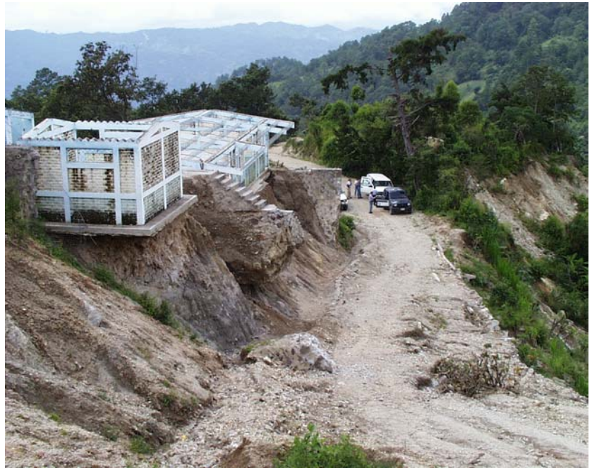
Figure 3. View of the El Pinar landslide and the abandoned school. A new road has been graded across the head of the landslide, which slid into the valley of the Río La Palma o Las Pozos on the right. Future movements on the landslide will likely disrupt the new road
