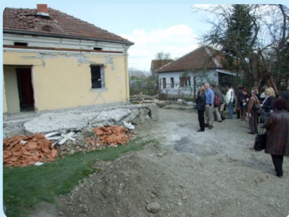
Effects of the Kraljevo earthquake in 2010 More than 16,000 buildings and houses were damaged. Total damage is estimated at over €100million
