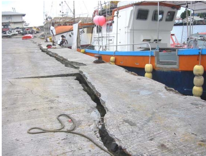
Figure 13: Tensional cracking due to movement of sheet piles toward the harbour. Repeated recession of floodwaters eroded a chasm beneath the offset concrete slab. Photo: DLF (GSC), 25 Jan 2005.
