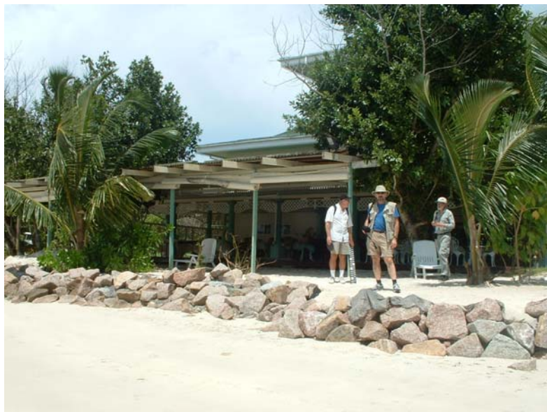
Fig. 73: Palm Beach Hotel, Grand Anse, Praslin. Note the low granite rip rap that supposedly provides defense against waves. The natural berm is gone and the coast is constrained. Photo: JS (GSC), 28 Jan 2005.
