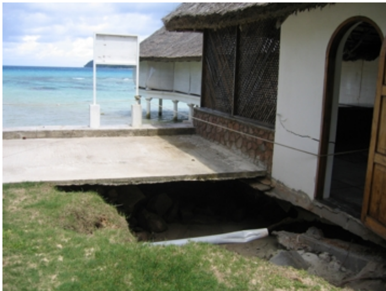
Fig. 63: Southwest side of pier restaurant showing erosion of foundation and partial collapse. Several of the piers of the structure in the background have rotated out of plumb. Photo: LEJ (GSC), 29 Jan 2005.
