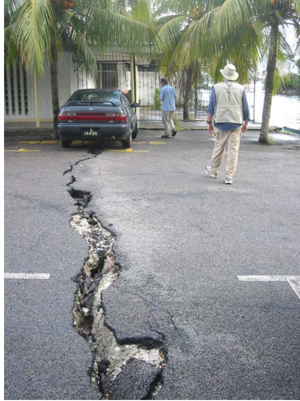
Fig. 15: Lateral spread failure intersecting building. Photo: DLF (GSC), 25 Jan 2005.
