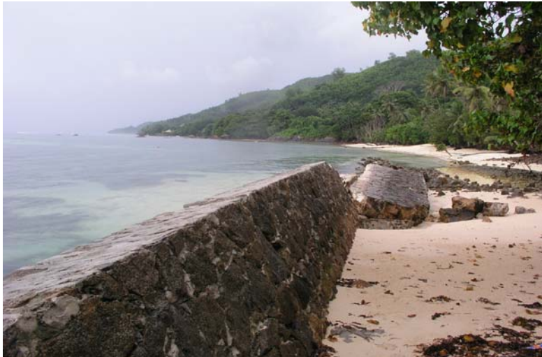
Fig. 32: Seawall that was damaged during the tsunami event just to the north of the profile. Photo: JVB (GSC), 25 Jan 2005.
