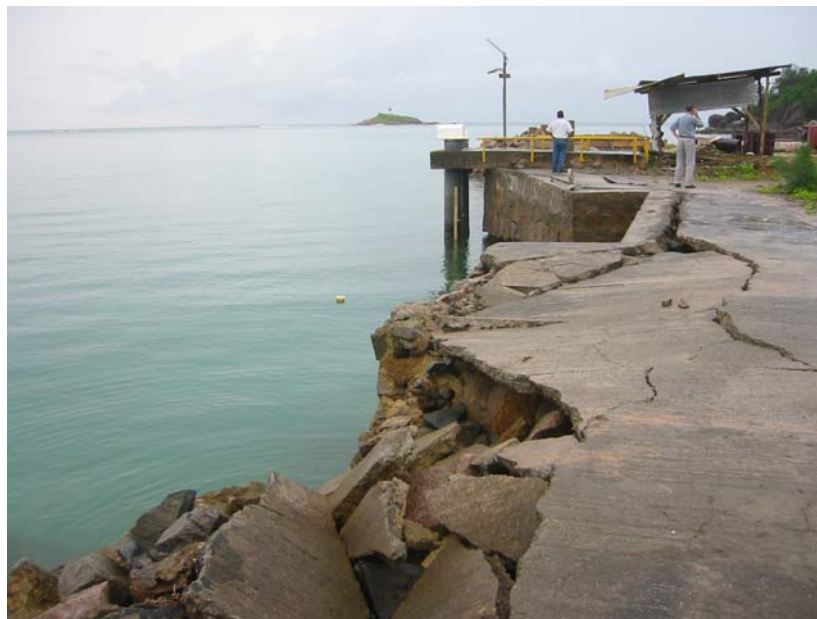
Fig. 17: Tide-gauge stilling wells and staff, showing structural damage to the wharf at the outer end of the jetty. Photo: LEJ (GSC) [DLF camera], 25 Jan 2005.
