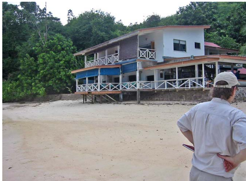
Fig. 24: Fairlyland Hotel. Highest tsunami water level reached to approximately the top of the railing along the first floor. Note the location of the building on the beach. A former beach berm has been removed and replaced by a low seawall. Photo: DLF (GSC), 24 Jan 2005. See also cover photo.
