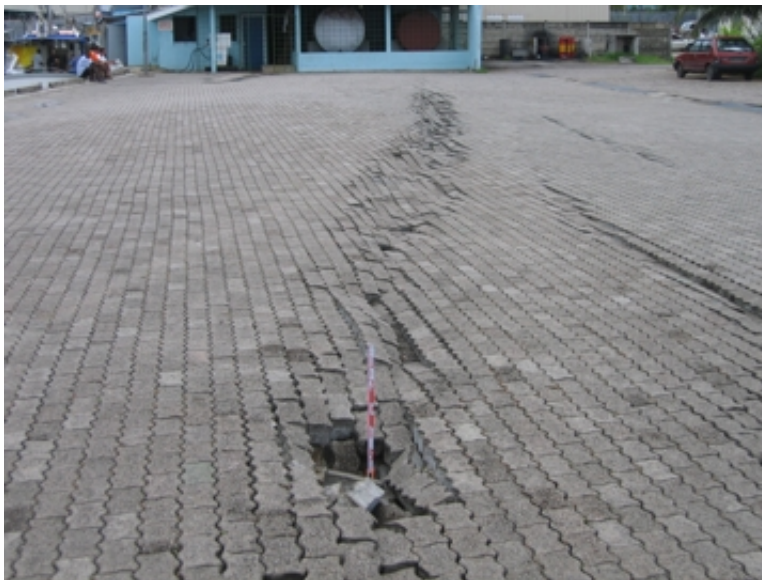
Fig. 14: Fissures created by dragging of anchor wall seaward. Adjacent sub-parallel cracks were caused by additional spreading of fill inboard of anchor wall (colour divisions on scale 10 cm). Photo: LEJ (GSC), 25 Jan 2005.
