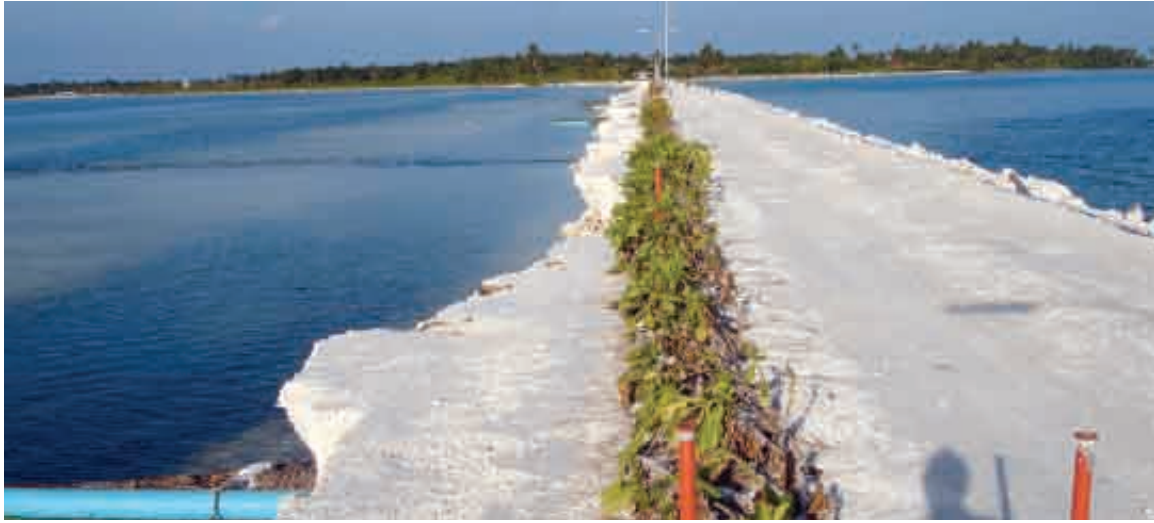
FIGURE 4.15: The causeway between Kaddhoo and Fonadhoo showing extensive erosion on the inside (left) caused by the formation of scour pits.
