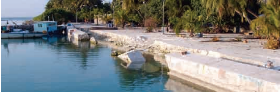
FIGURE 4.23: Collapse of the harbour wall at Vilufushi.
