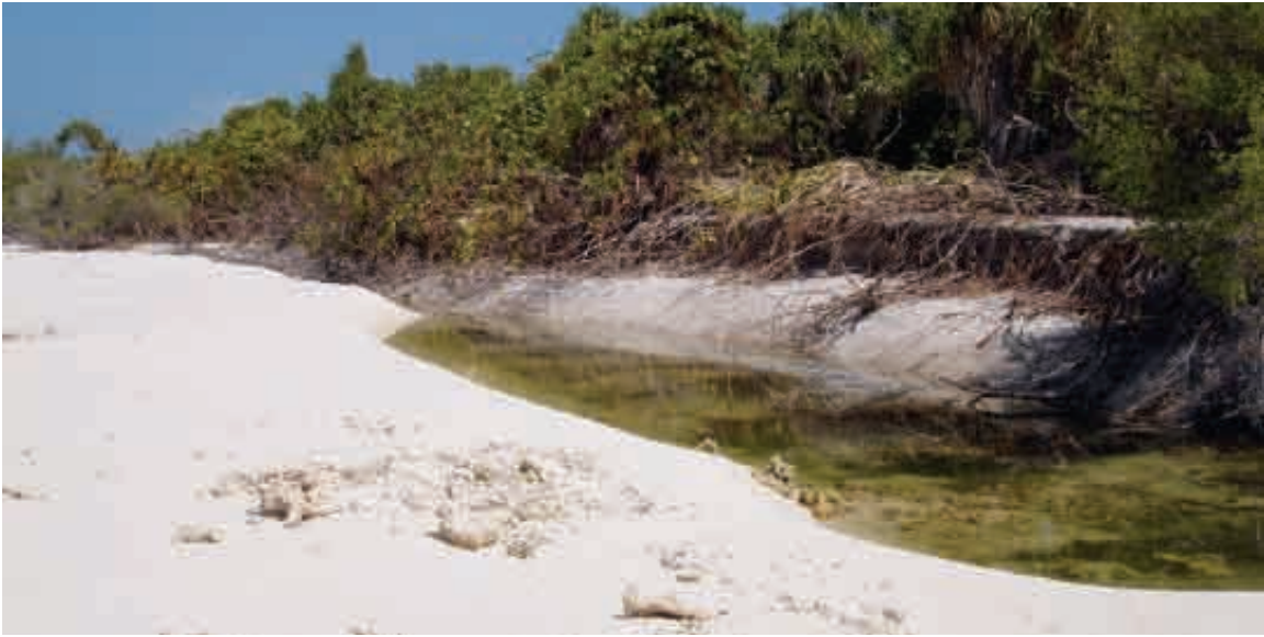
FIGURE 4.11: Scour pits on Uvadhevifushi.
