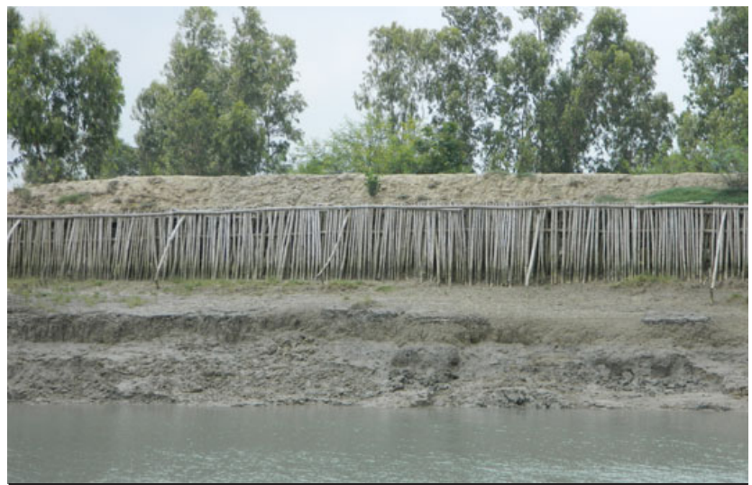
Eroded River Embankments in the Sunderbans, Concern Worldwide, Photographer : Jyotiraj Patra.
