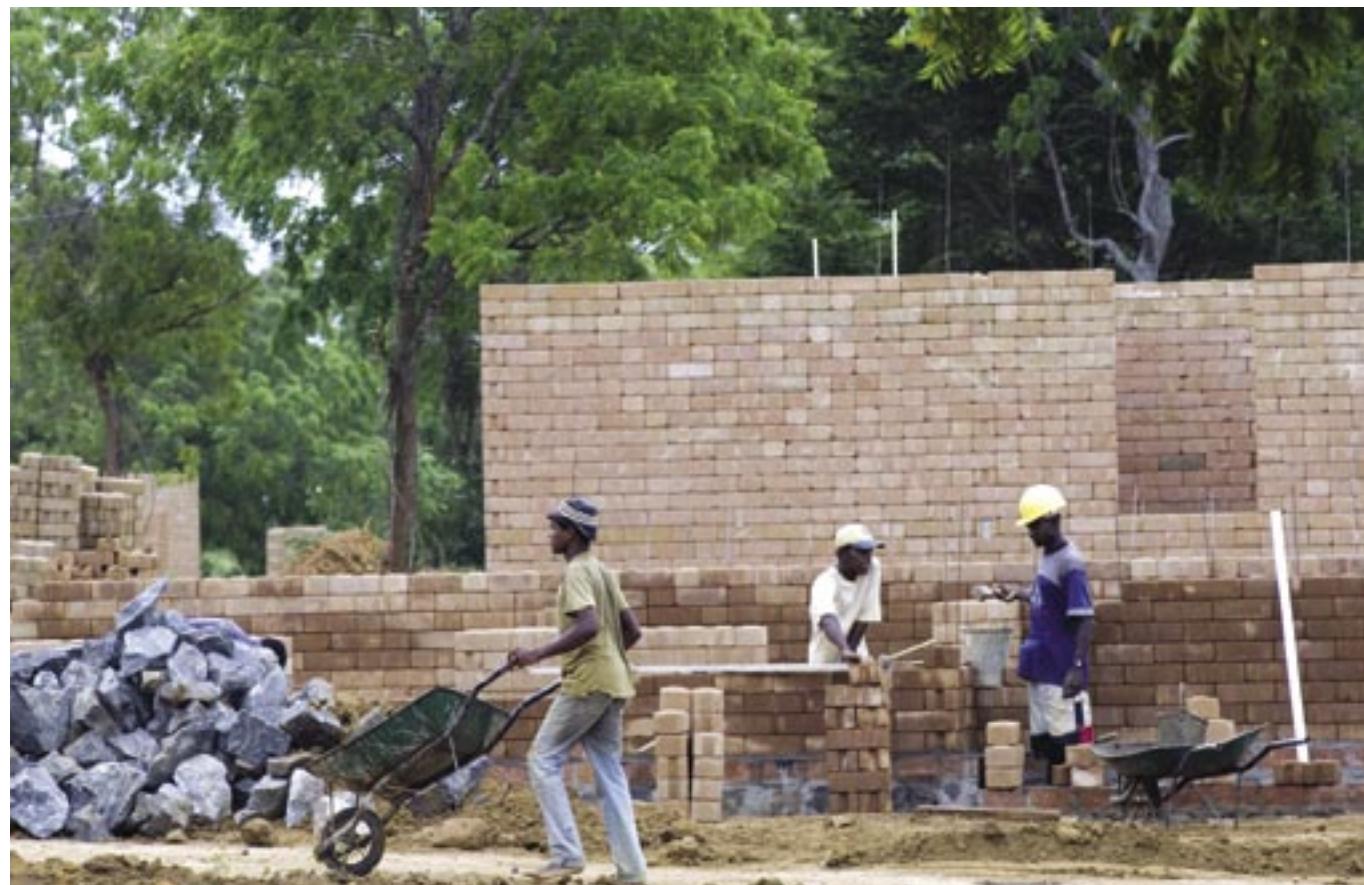
Families involved in constructing their own homes were more satisfied than those in settlements
