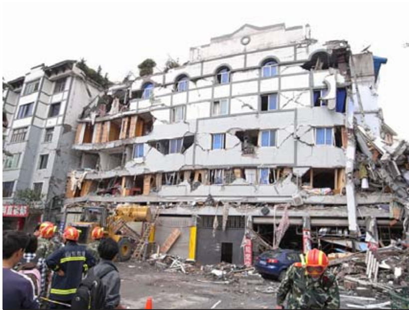
A collapsed building in Dujiangyan, close to the epicentre of the 2008 Sichuan earthquake. (Source: http://www.sustainablechina.info/2009/01/29/did-chinas-dams-trigger-the-sichuan-earthquake/ )
