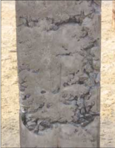
Honeycomb in column concrete
