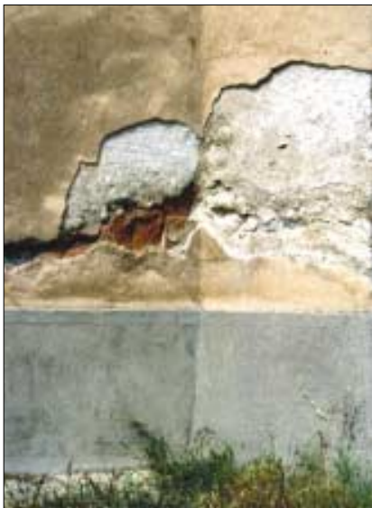
Cement plaster at the bottom leads to further rise of rising damp and salt crystallization
