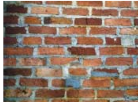
Under burnt bricks will not have enough strength and weather over a period of time
