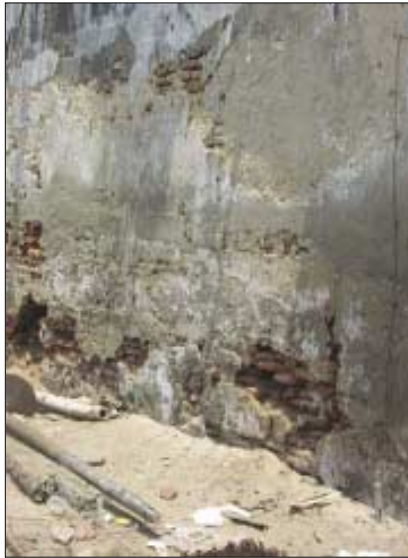
Rising dampness and salt crystallization leads to weathering
