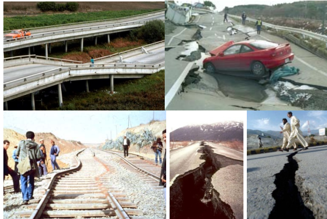
Destruction of bridges, roads and railways
