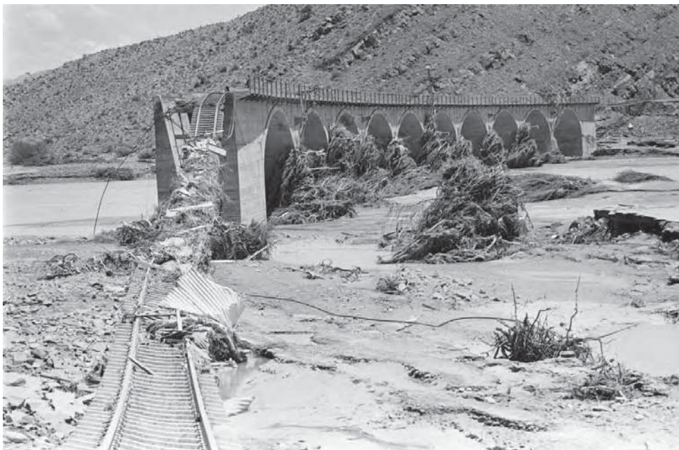
Damage sustained by the railway bridge following the 1981 Laingsburg floods when the Buffels River flooded, claiming more than 100 lives.
