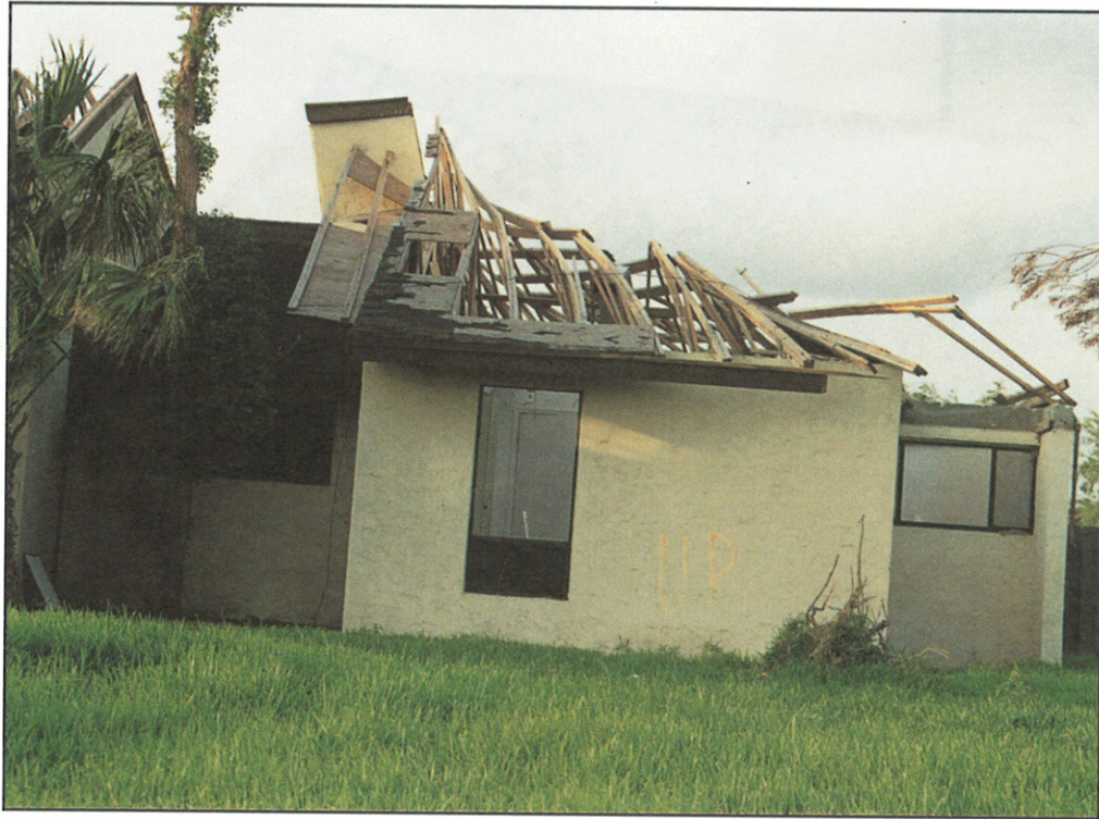
FIGURE 14. Roof structure failure due to inadequate bracing.
