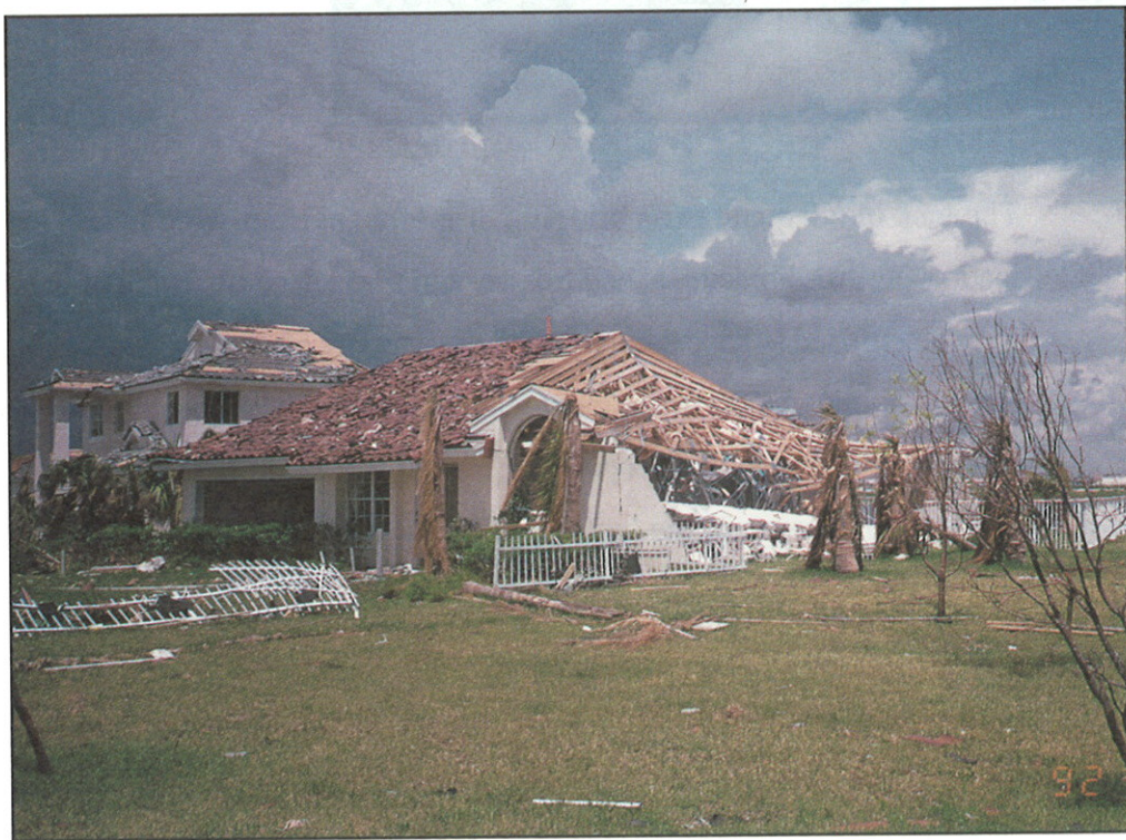
FIGURE 13. Roof structure failure due to inadequate bracing.
