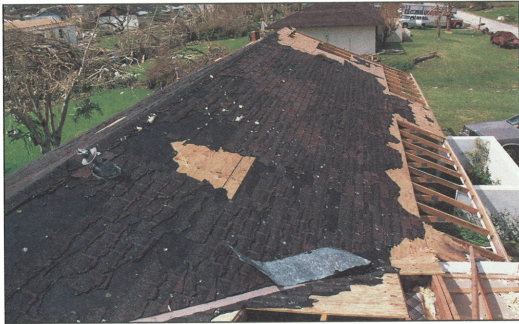
FIGURE 30. Composition shingle and underlayment failure.
