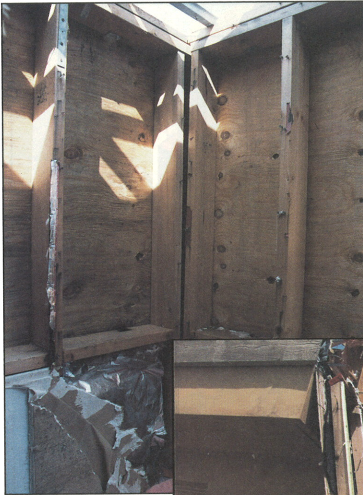
FIGURE 59. End column/corner post missing from wall.
