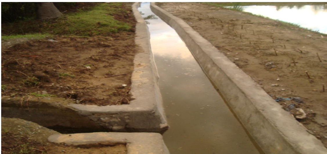
Fig. 3. A drainage system constructed at Mieuruk village in Aceh Besar to avoid impact of inundation.
