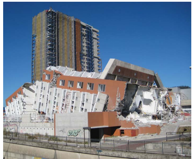
Figure 1. Building Collapsed when the magnitude 8.8 earthquake struck Chile in February 2010, © AIR Worldwide 2010
