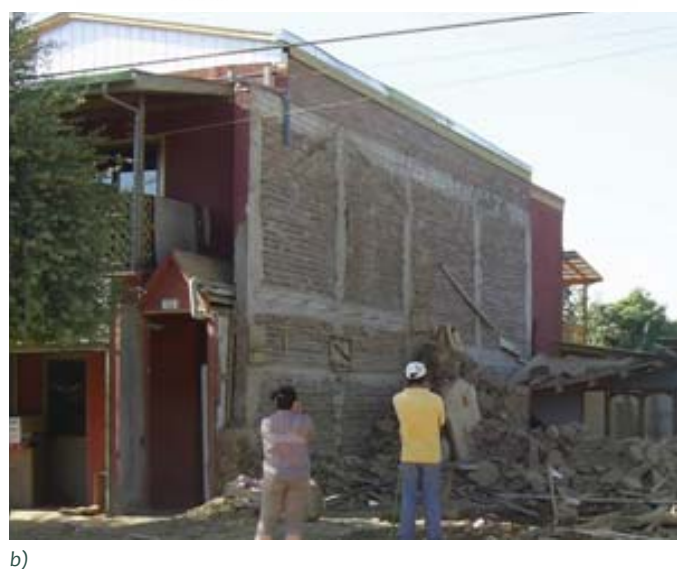
Figure 3. Confined masonry buildings: a) key components, and b) good performance of confined masonry in the 2010 Maule, Chile earthquake (M.O. Moroni Yadin).
