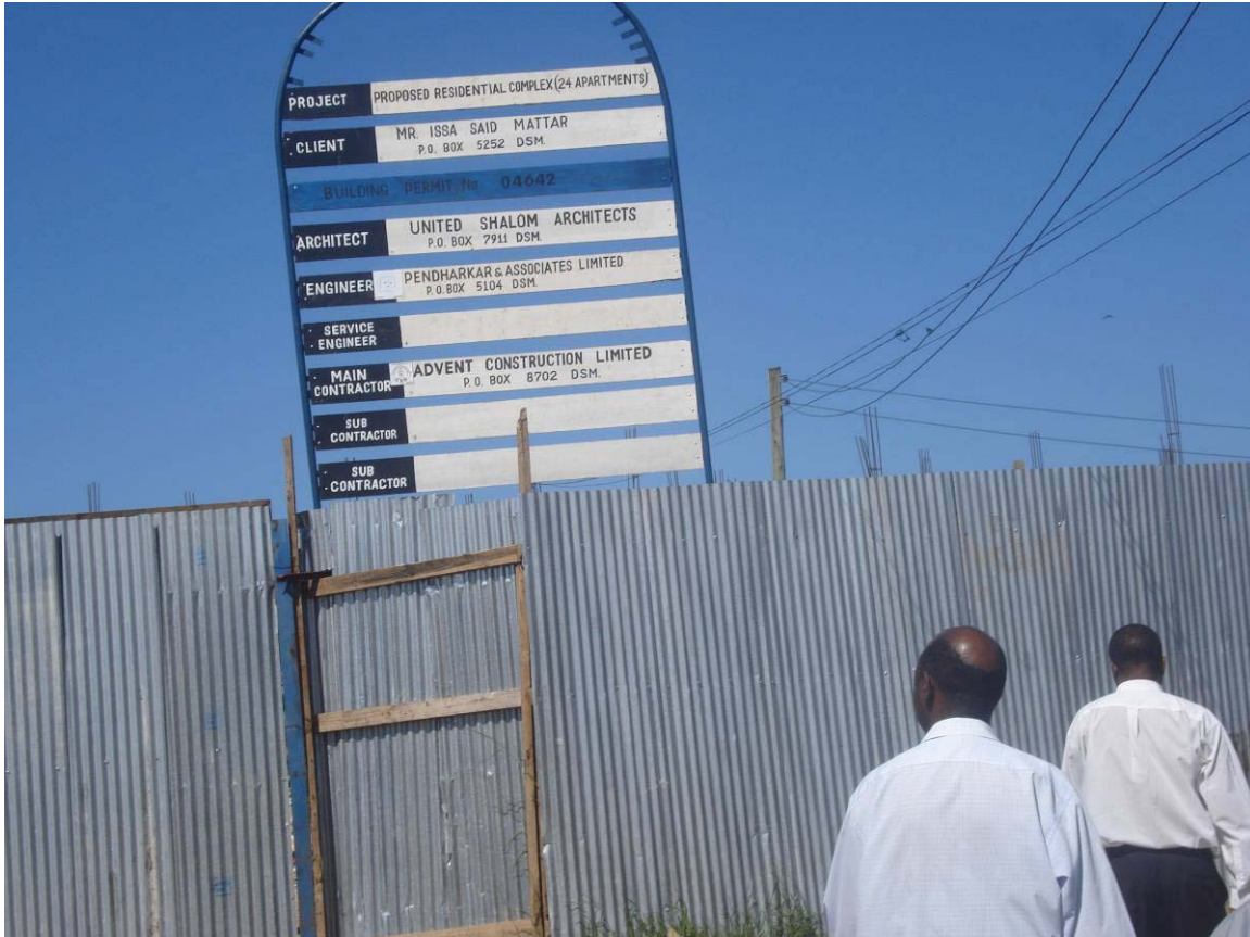
Plate 3.1: Fenced site in which 24 residential apartments are being constructed within the wetland
