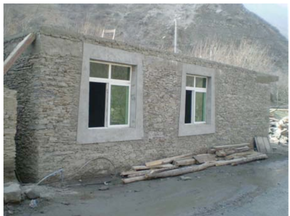
Housing reconstruction by traditional masonry construction method of the Qiang people (In Lixian County, December 25, 2008)
