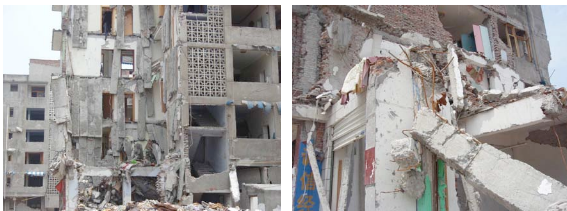
Collapsed mid- and high-rise housing complex in Dujiangyan City (in June 2008)
