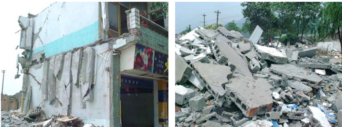
Damage on houses in the center of Zhundao Town of Mianzhu City (Right: Buildings were lost their original form in this district). The photos were taken in June.
