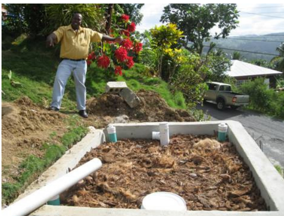
Accessible technology solutions, such as this wetlands filtration system, are being constructed in Saint Lucia as part of an overall approach to managing wastewater in a changing climate. (Photo by Donna Spencer).
