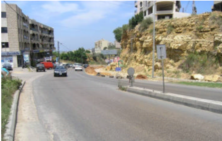
(a) Toppling of rocks triggered by heavy precipitation blocked the Mansourieh main highway partially (Mount Lebanon)
