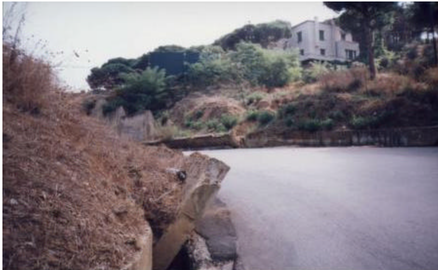
Figure 23. Bad construction of retaining walls aggravating the risk of landslides
