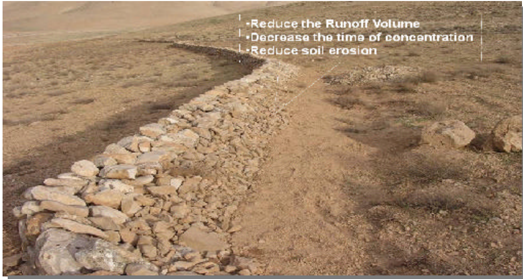
Figure 22. Stone wall structures to reduce the adverse effects of devastating floods in El Qaa watershed (Lebanon) (GTZ and ACSAD, 2008)
