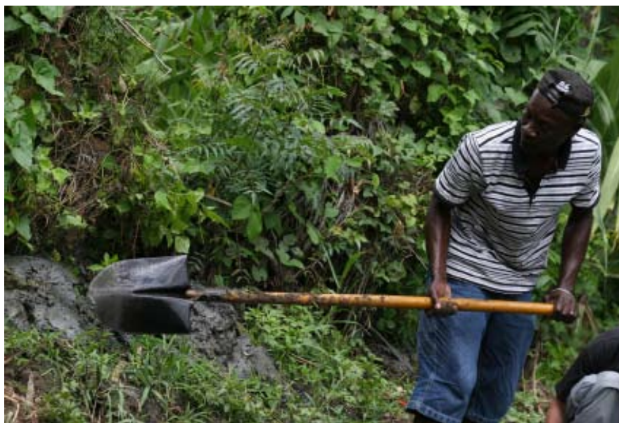
Cash for Work. In its post-emergency responses, Oxfam is assisting community resident to dig ditches which alleviate the impact of floods – and help with irrigation during dry periods or droughts. © Bernard Cherelus/Oxfam
