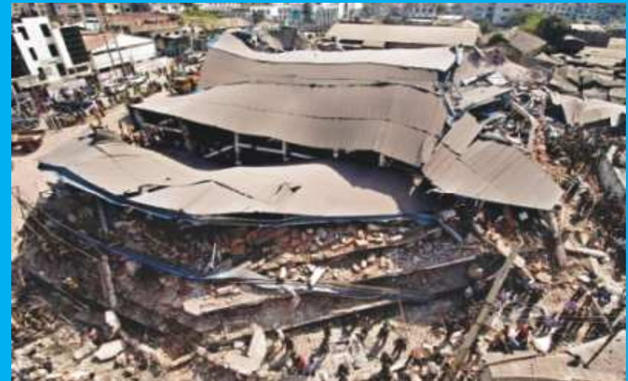
6 story building collapsed- died 21, 25/02/2006
