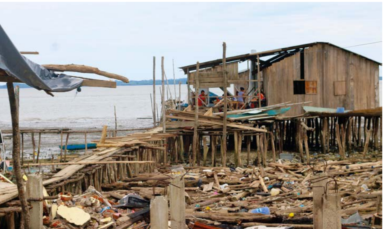
Debris at the fishing village of San Jose de Chamanga, Ecuador, a few kilometres away from the M7.8 epicentre of April 2016. Photo: NORCAP/IOM/Fernanda Baumhardt, June 2016
