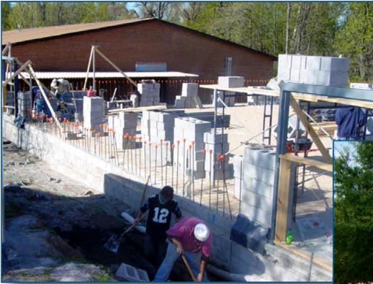
The College Station Elementary School shelter during construction (left) and the completed stand-alone shelter (right). (SOURCE: WAPDD)
