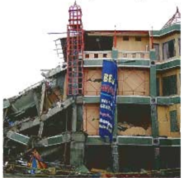
Earth Quake Damage, Leveling Shops
