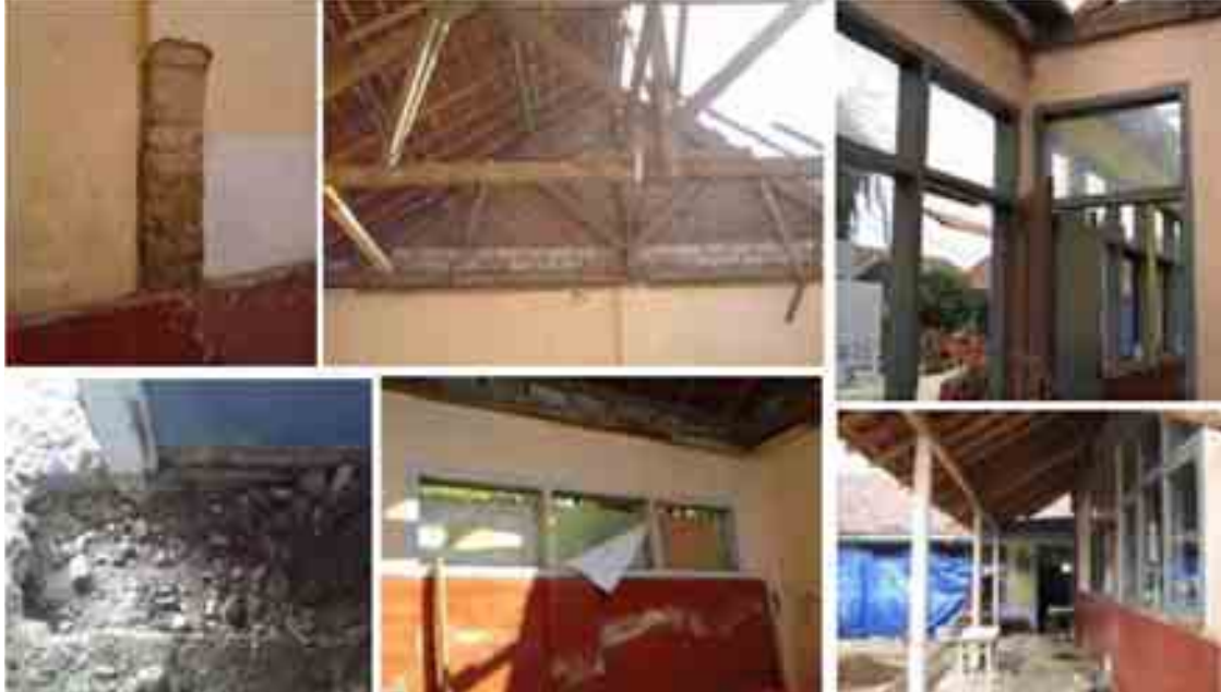
Figure 81: Existing structural condition of SD Cirateun Kulon II
