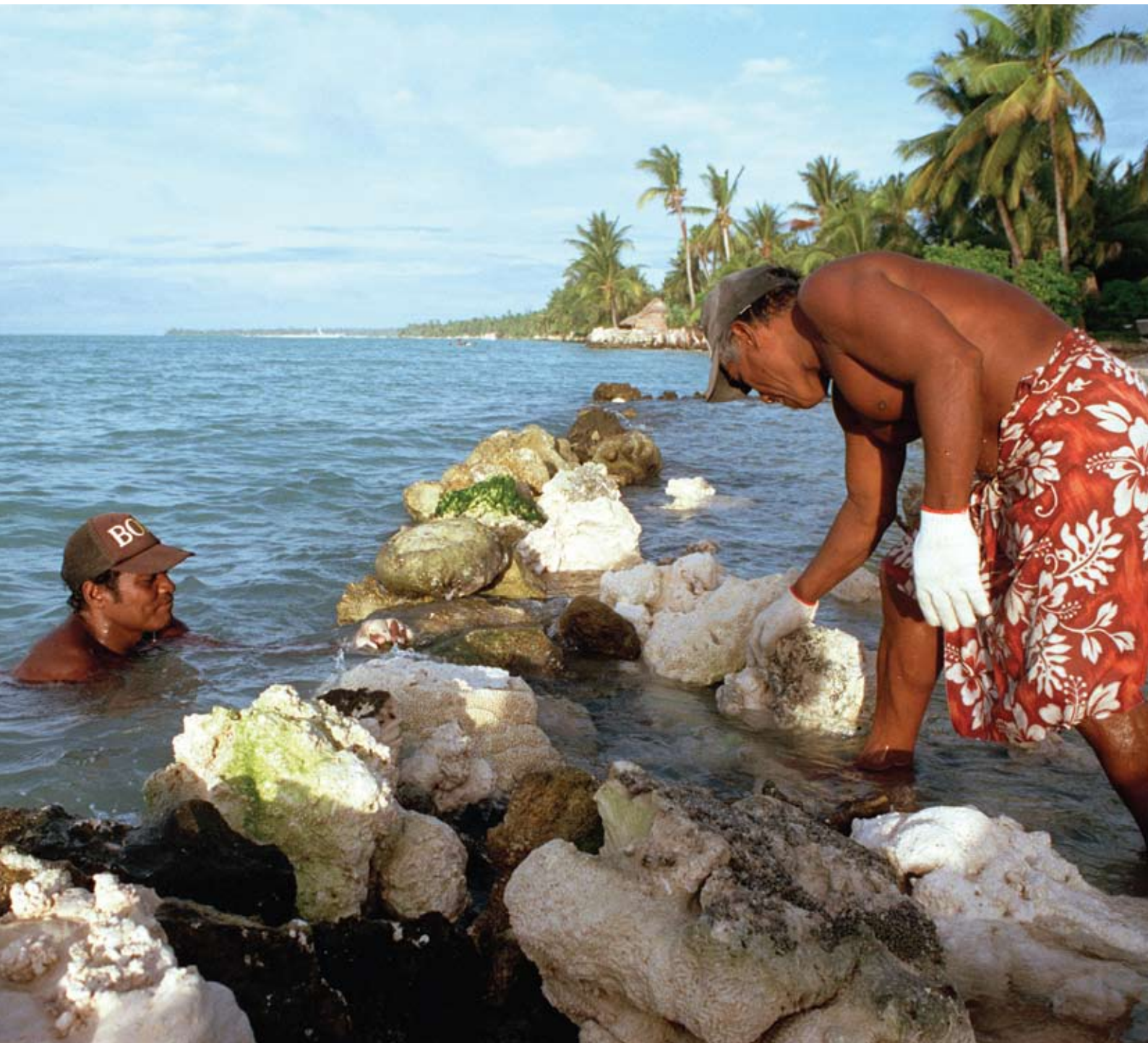
A coral wall intended to break the swell of king tides and storm surges is being constructed in order to protect residents in Tarawa, Kiribati.
