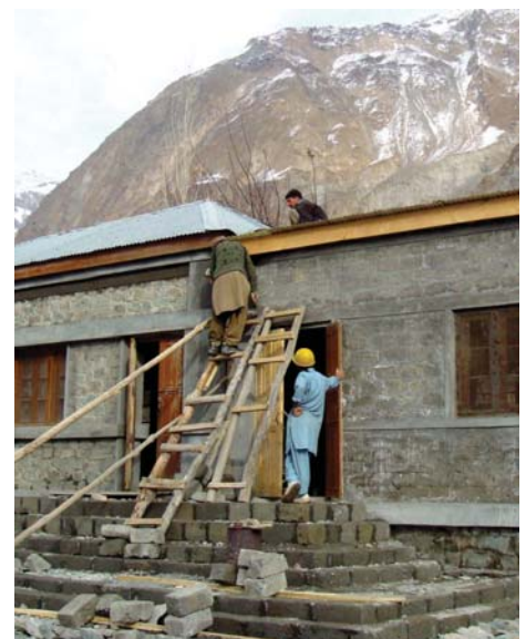
Seismic retrofitting in progress at DJ Primary School, Hasis, Ghizar, Northern Areas, Pakistan 2008. The local community is actively participating in the retrofitting work
